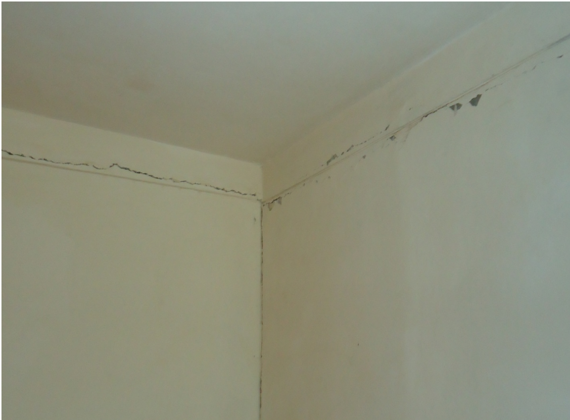
Figure 4:7: Case study02 actual damage view photo
