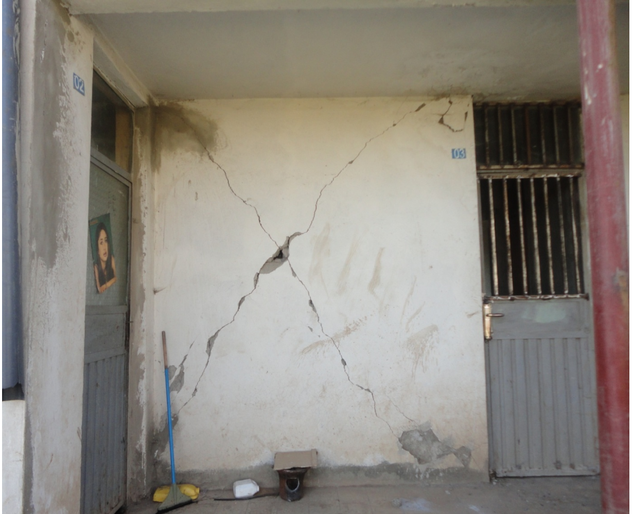
Figure 4:2: Case study 01 actual damage photo
