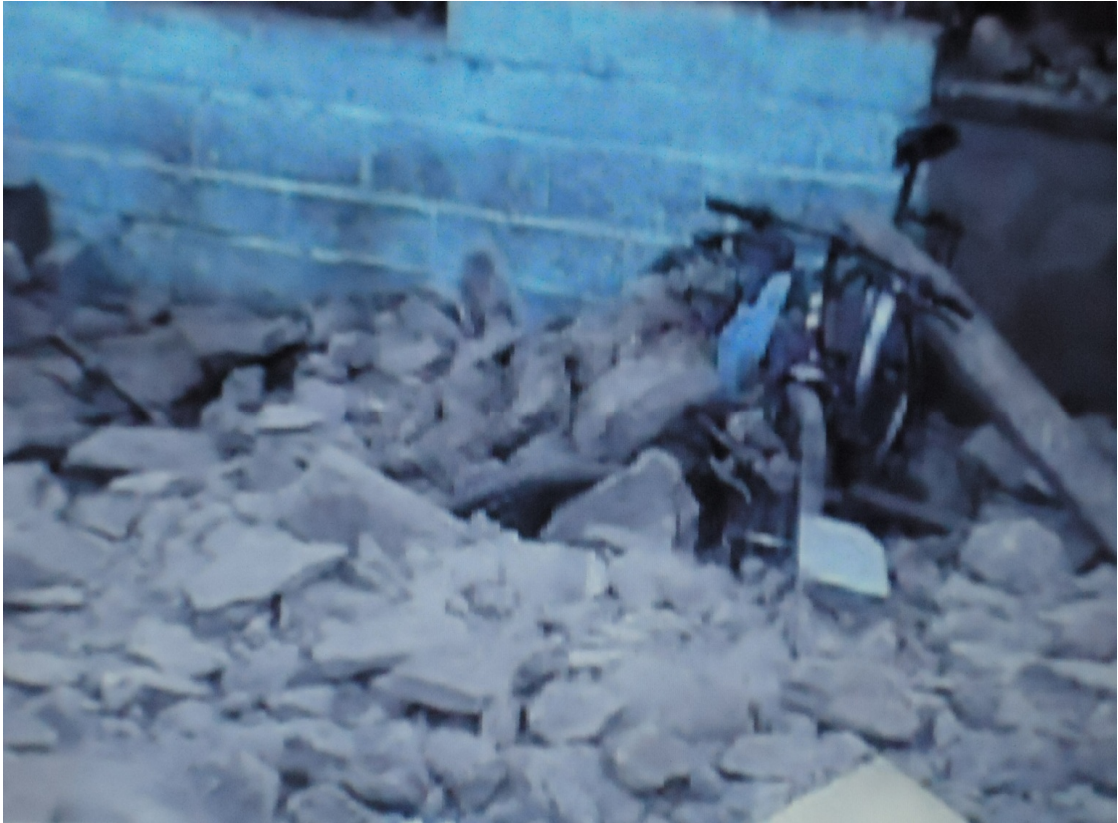
Figure 4:15: Damage photo of case study 05
