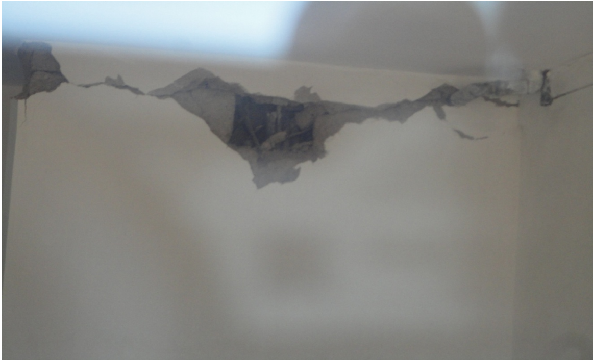
Figure 4:10: Actual damage view photo of case study 03 building
