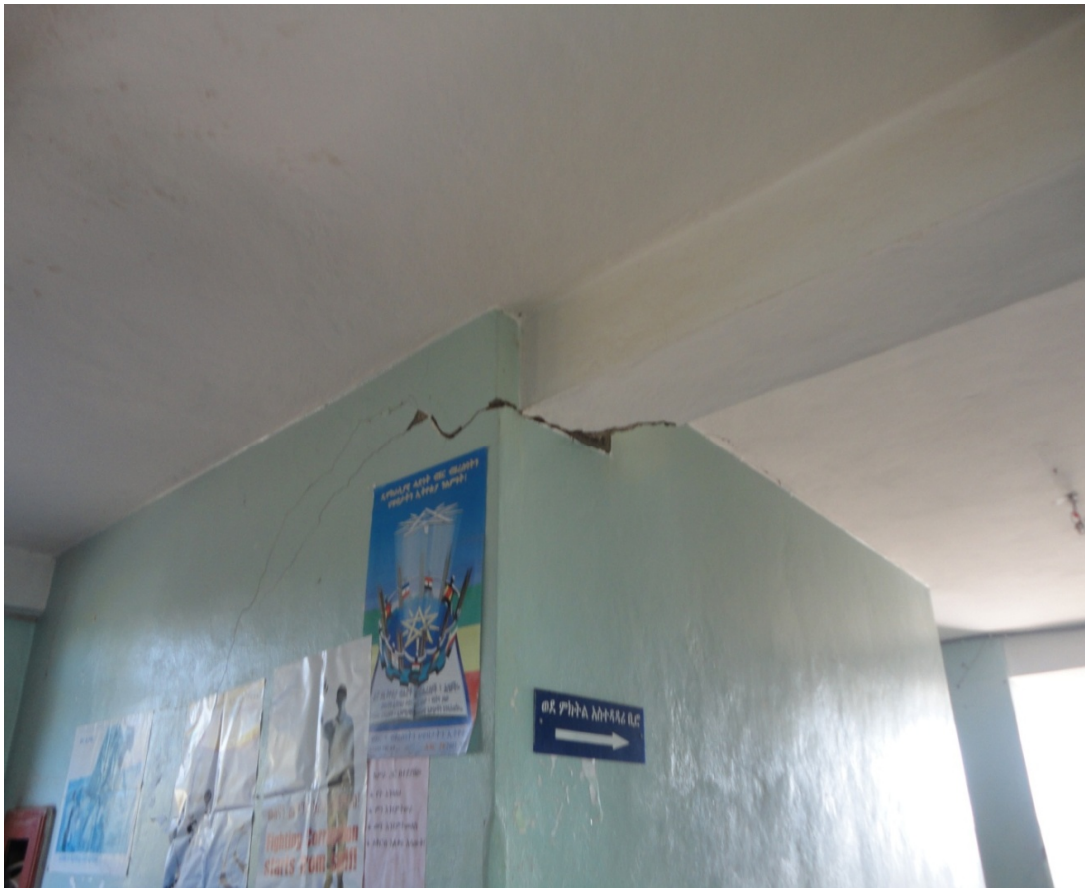
Figure 4:9 : Actual damage view photos of case study 03 building
