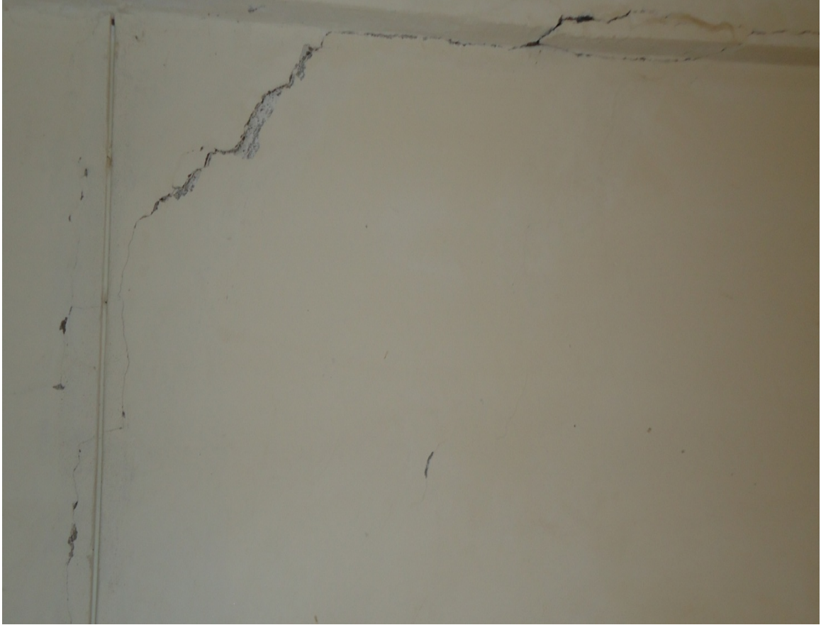
Figure 4:6: Case study02 actual damage view photo
