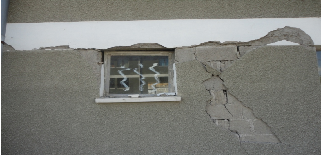
Figure 4:4: Case Study 01 actual damage photo
