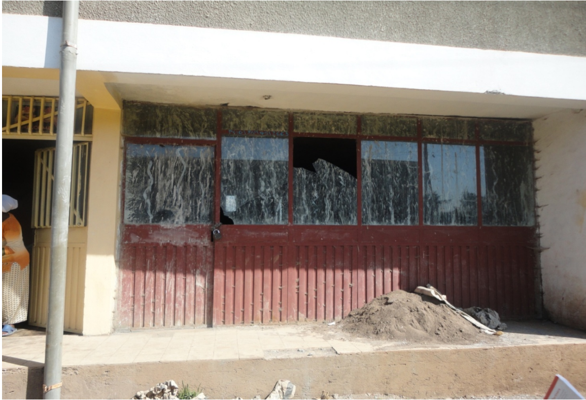
Figure 4:3: Case study01 damage view photo
