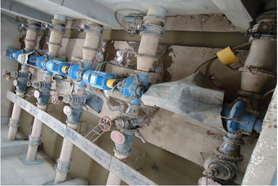
Figure 3. 1 Pump station for Kawa command area
