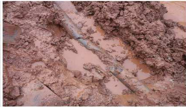
Longitudinal split on a polyvinyl chloride pipe.
