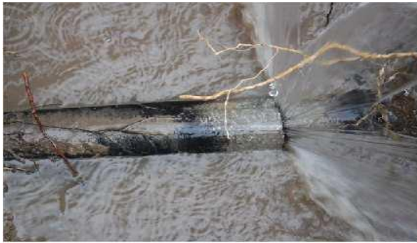
Circumferential break on an asbestos cement pipe.
