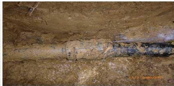
Joint failure (disconnection or gasket failure) on an asbestos cement pipe.
