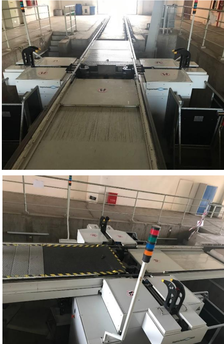
Figure 3.6-Underfloor wheel lathe in AALRT (Courtesy of AALRT RS Depot)
