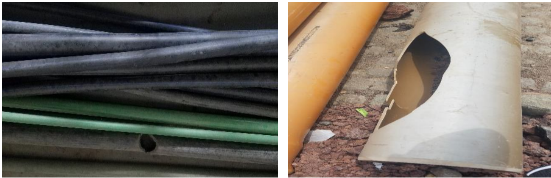
Figure 12: Observed quality defect Pin Hole
