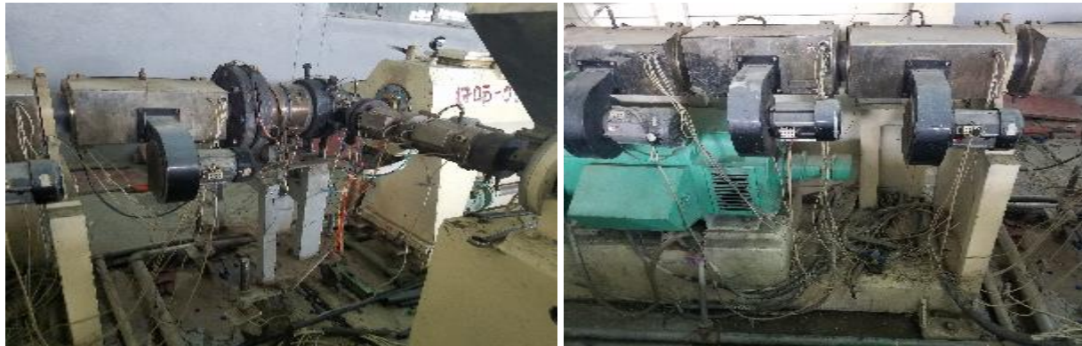
Figure 10: Defect occurrence in Electrical Power Interruption
