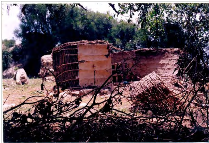
Fig. 1.5 A house damaged by the rolling of rocks in 2002
