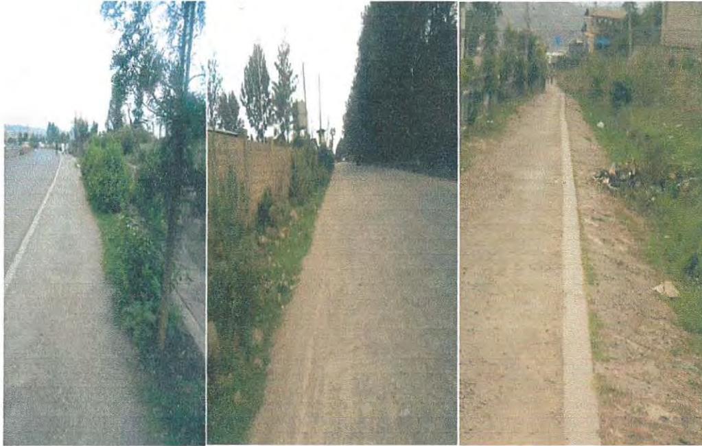
Picture 5: road sides those are not clean with shrubs, hidden and cluttered areas
