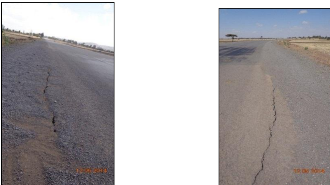
Figure 3.5: Road Failures near to Pavement Edge on shoulders (Severely damaged section around km 14 +000 in Modjo-Ejere Road segment)
