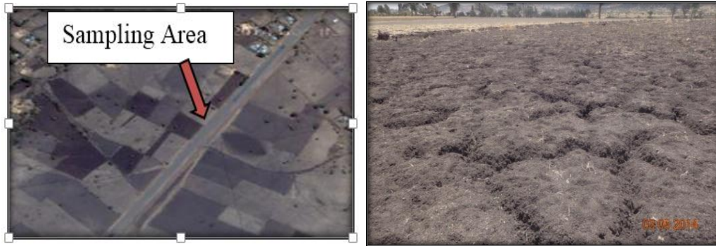
Figure 3.4: Expansive Soils in Modjio-Ejerie Road around km 14+000 where pavement failure observed.
