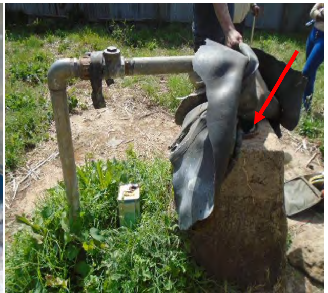
Plate 5.8 Well head protection that is not capped in Bui which is 350m deep
