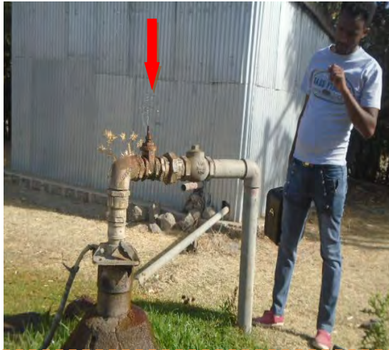
Plate 5.2 Water flowing through coupling in Asgori
