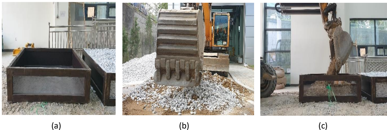
Figure 5.1. Construction of ballast boxes. (a) Build wooden box (b) Mix with fouled materials (c) Construct ballast layer [42]
