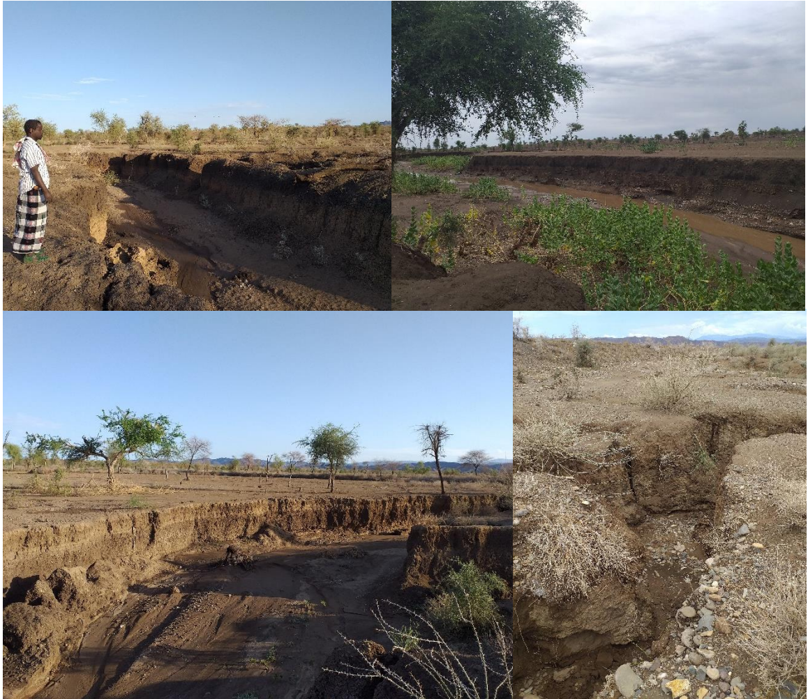
Figure 13: Eroded sites where Weirs are not constructed
