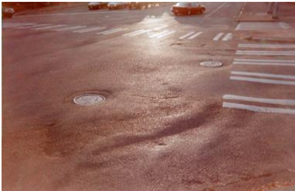
Figure 2.7 Shoving Type Surface Deformation in Flexible Pavement
