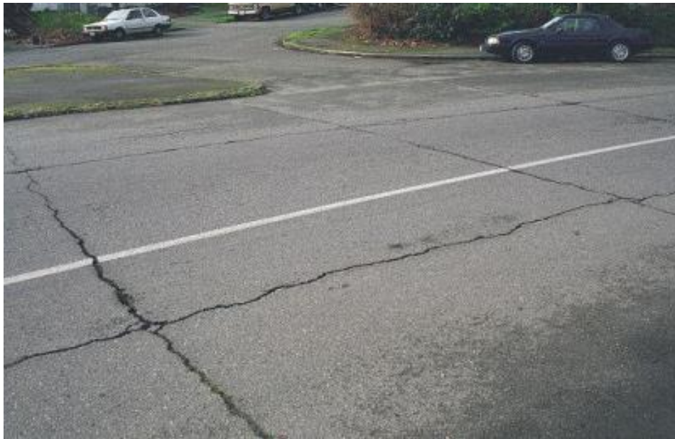
Figure 2.5 Reflective Cracking in Flexible Pavement
