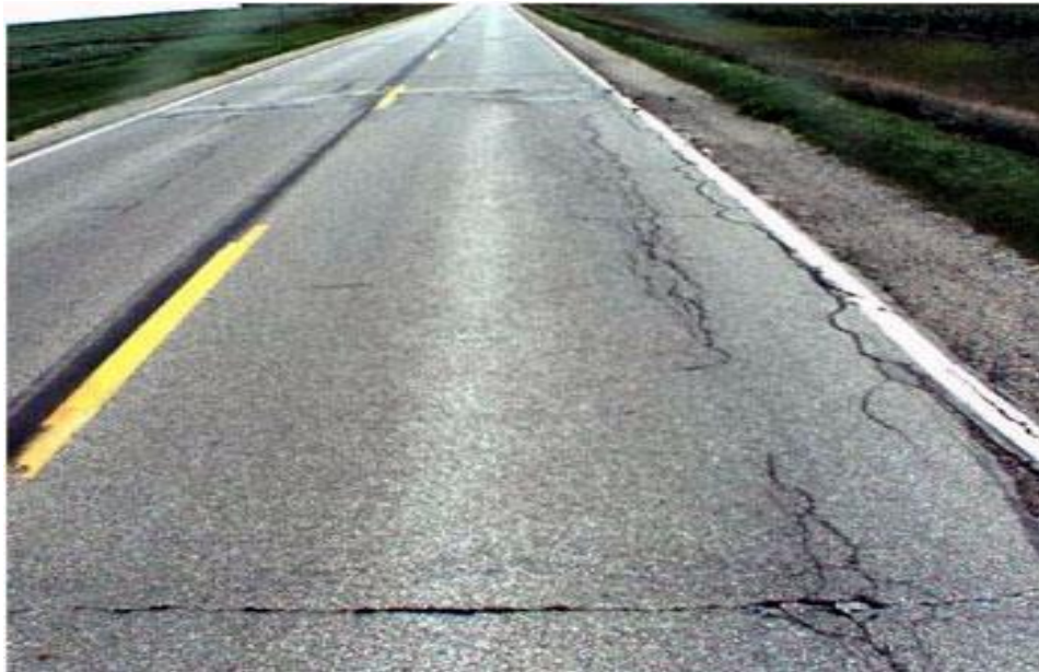
Figure 2.1 Fatigue Cracking in Flexible Pavement
