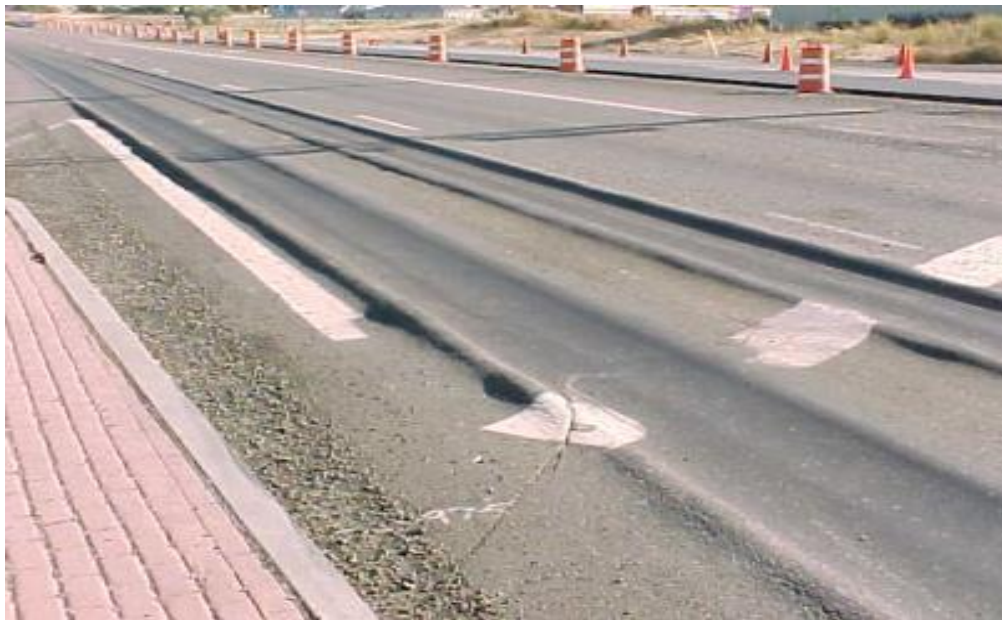
Figure 2.6 Rutting Type Surface Deformation in Flexible Pavement
