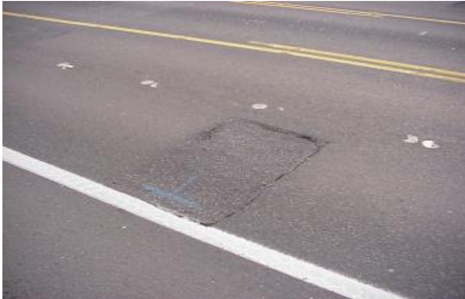
Figure 2.10 Patches Type Disintegration in Flexible Pavement
