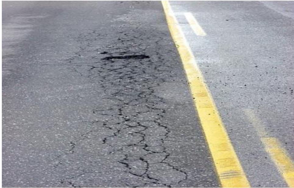
Figure 2.9 Potholes Type Disintegration in Flexible Pavement.
