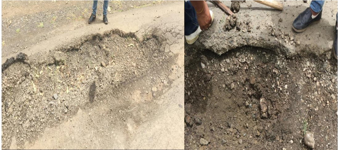
Figure 3.3 Representative Corrugation Type Damaged and their Samples (27/09/2010 E.C)
