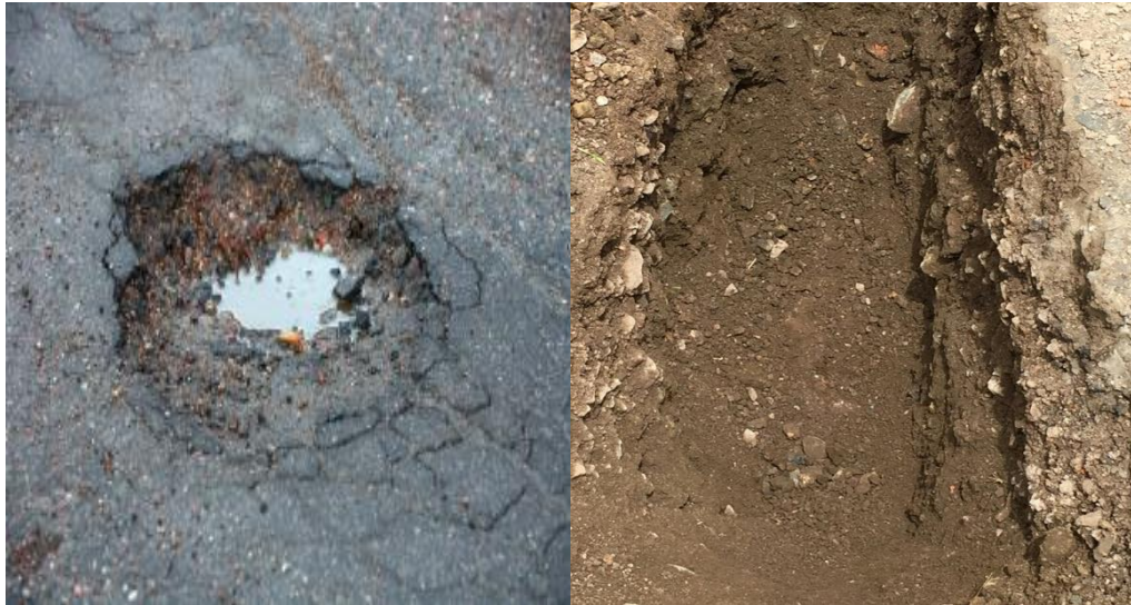
Figure 3.4 Representative Potholes Damages and their Samples (27/09/2010 E.C)
