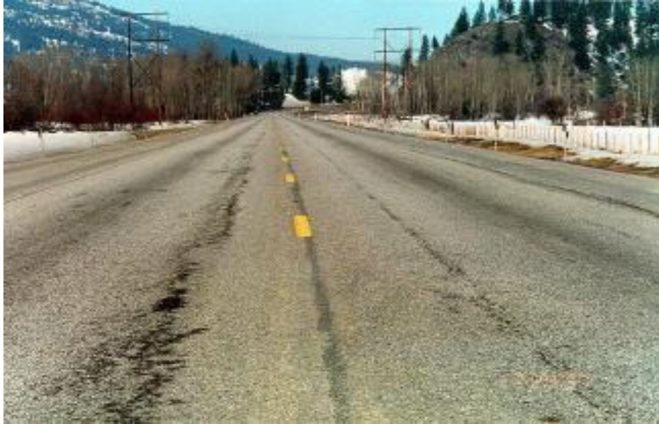
Figure 2.11 Raveling Type Surface Defects in Flexible Pavement
