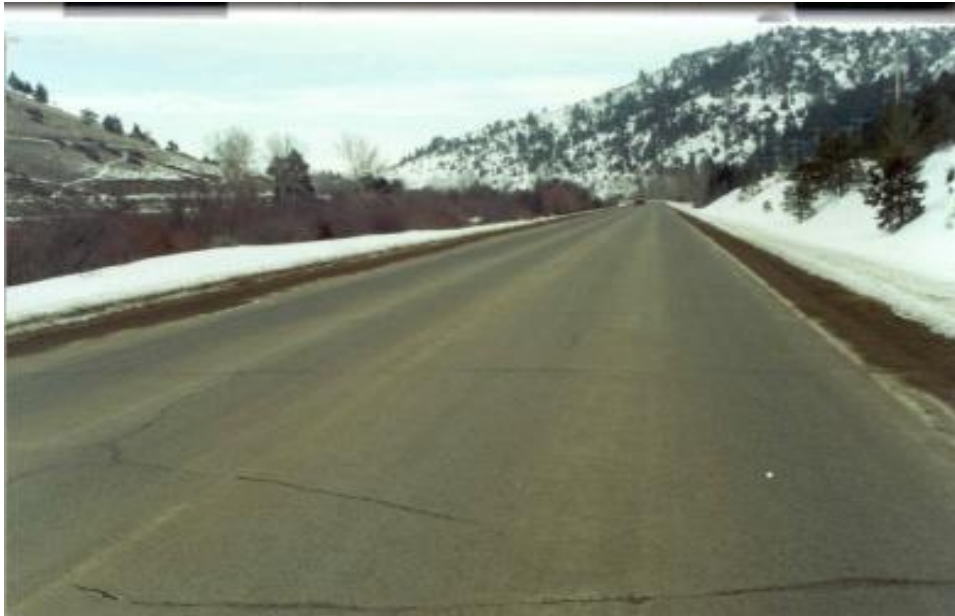
Figure 2.2 Transverse Cracking in Flexible Pavement
