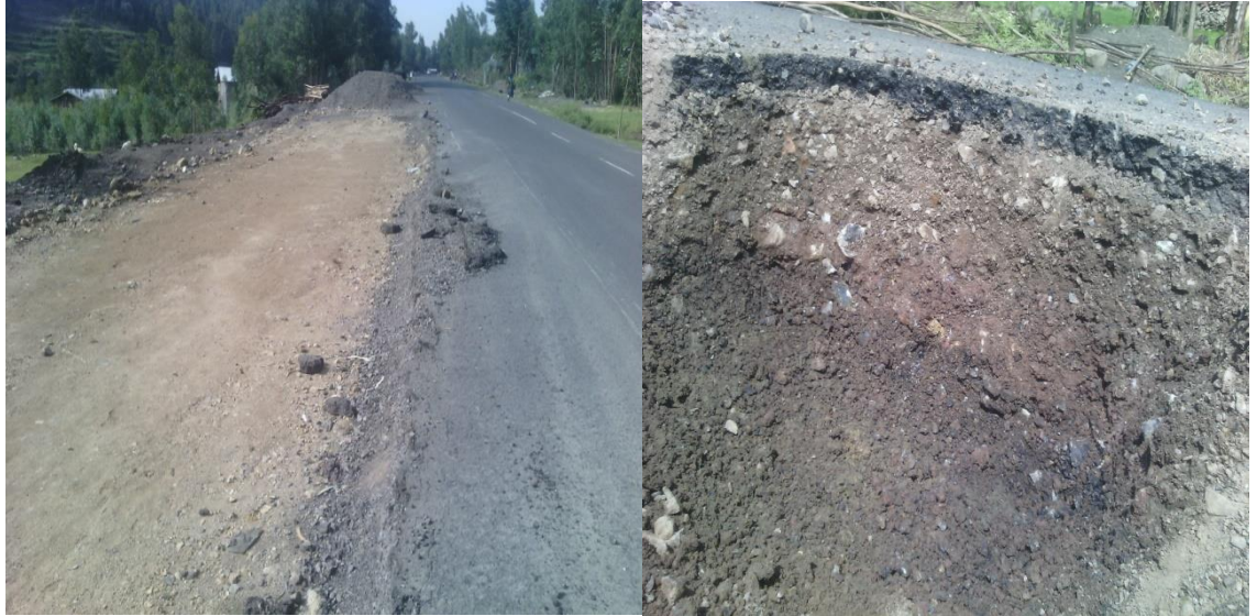
Figure 3.2 Representative Patched Damaged and their Samples (27/09/2010 E.C)
