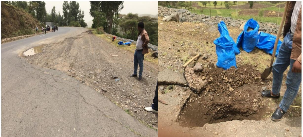
Figure 3.1 Representative Raveling Damage and their Sample (19/09/2010E.C)
