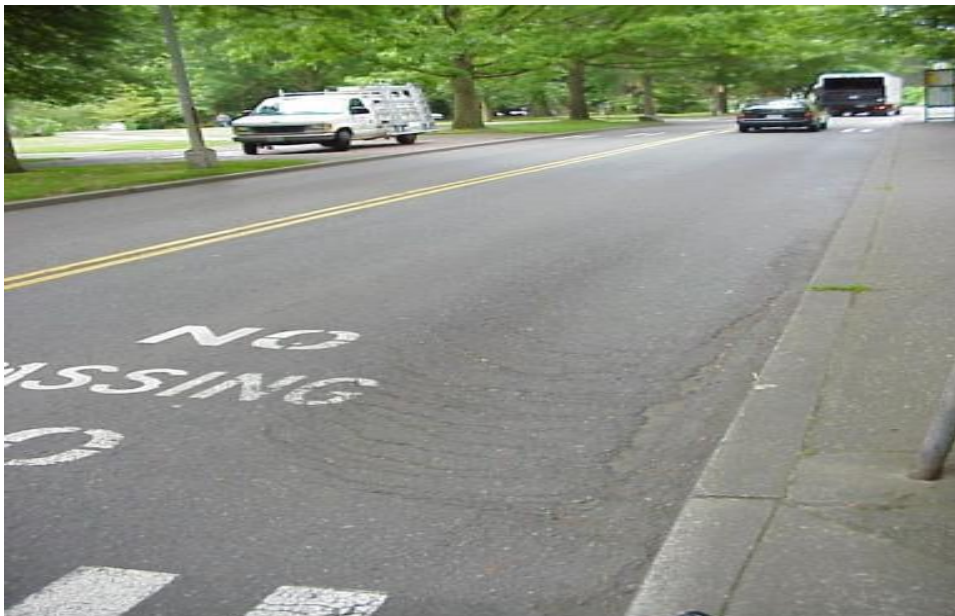
Figure 2.4 Slippage Cracks in Flexible Pavement
