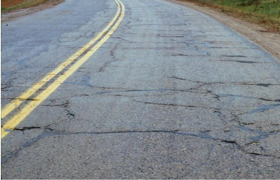
Figure 2.3 Block Cracking in Flexible Pavement
