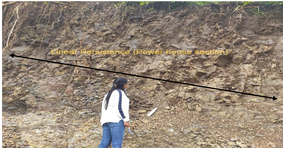
Fig 2.12: Persistence (Joint Length) of rock outcrop (Location: Project site, Proposed Power House section of the Tunnel Route)
