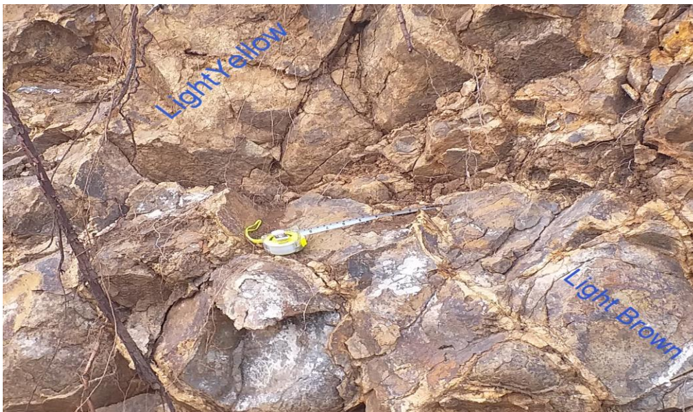
Fig 2.5: Highly weathered basalt based on color indication (Location: Project site, left of abutment proposed Dam section)
