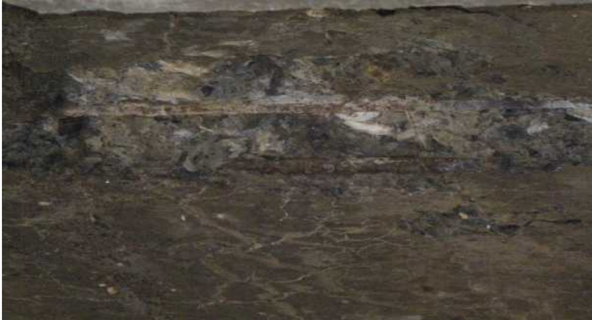
Plate 2.3.3: Rebar exposure due to peel off and delaminating
