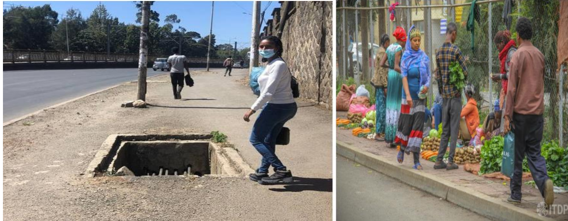
Figure 3.9 Example of Open Manhole in the Middle of Walkway and Street Vending
