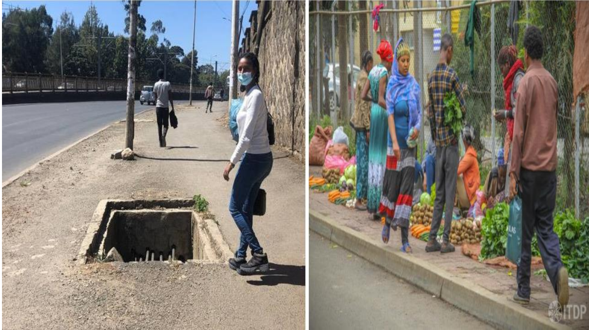
Figure 4.11 Example of Open Manhole in the Middle of Walkway and Street Vending Source: AATB, 2022
