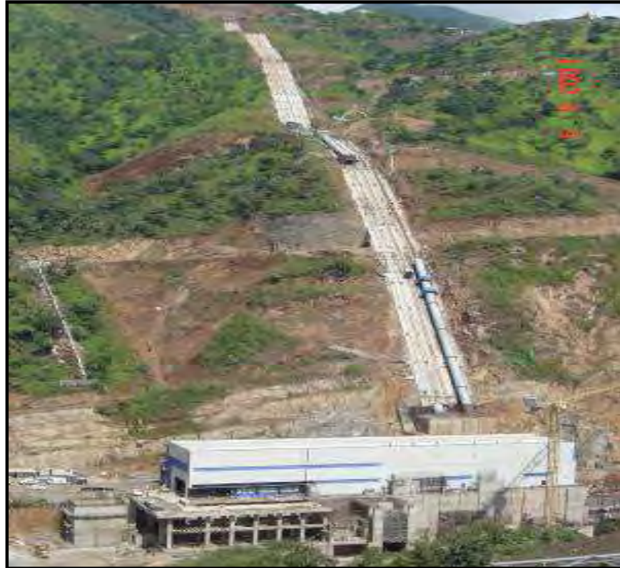
Figure 3-7 Photograph view of Gibe II power house and penstocks
