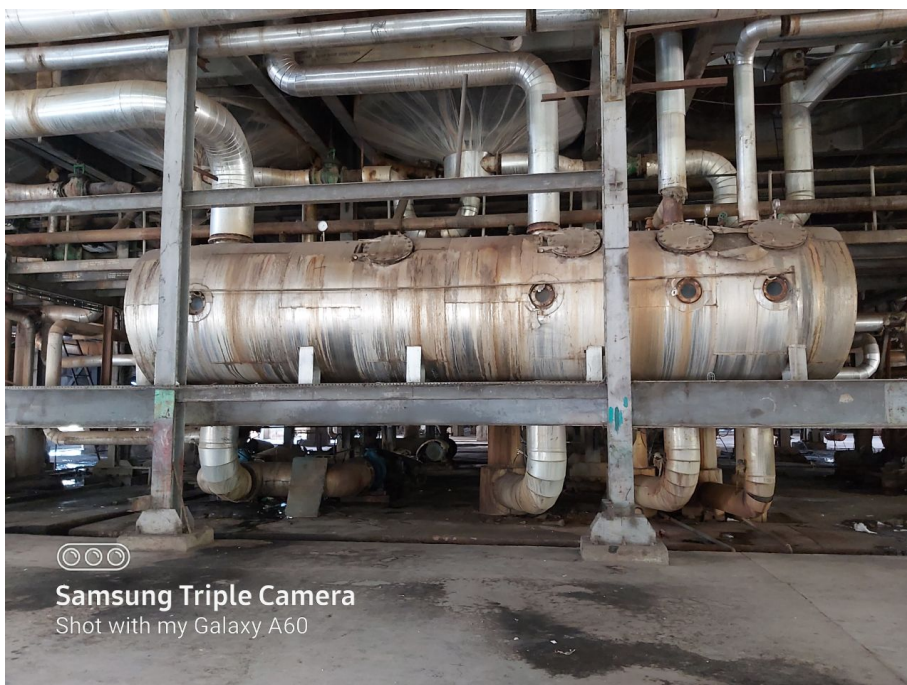
Figure 2.1: Woni /shoa sugar factory first effect evaporator condensate flash tank
