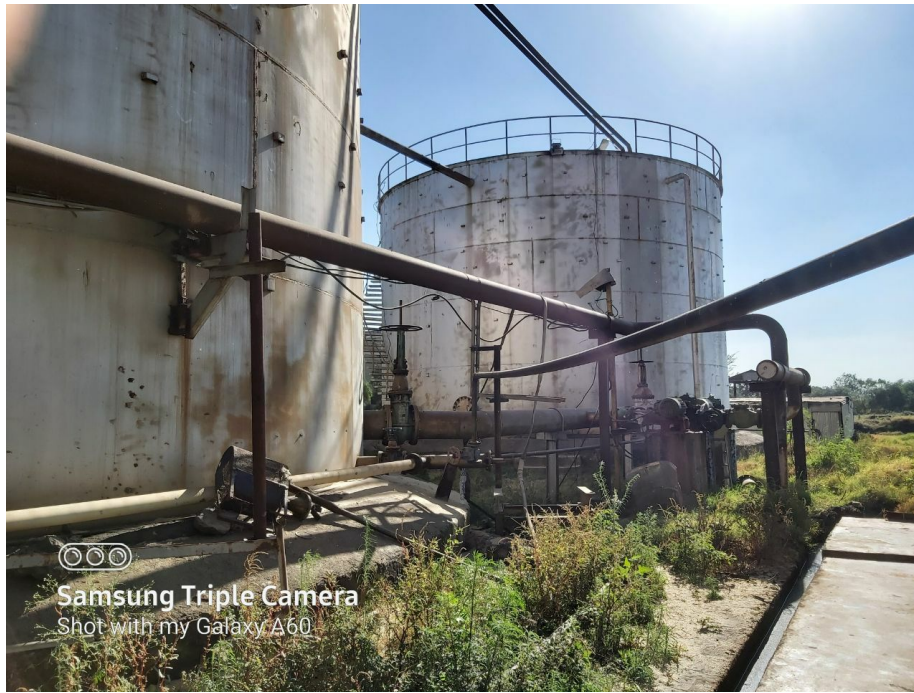
Figure 2.2 : Wonji/shoa factory surplus tank for condensate and make up water
