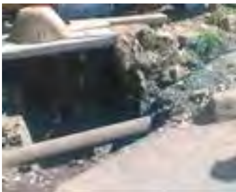
2 not well managed drainage
