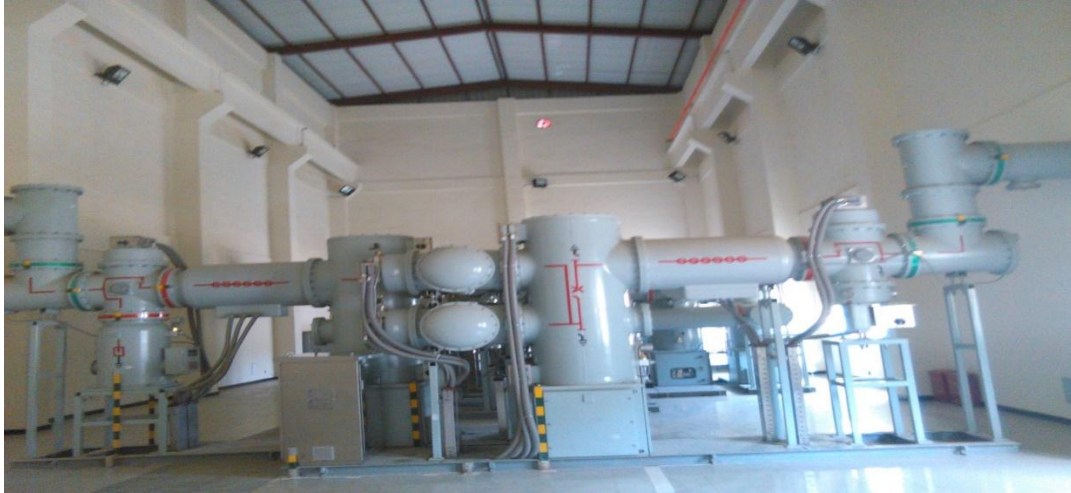
Figure 1.1 132KV gas insulated substation
