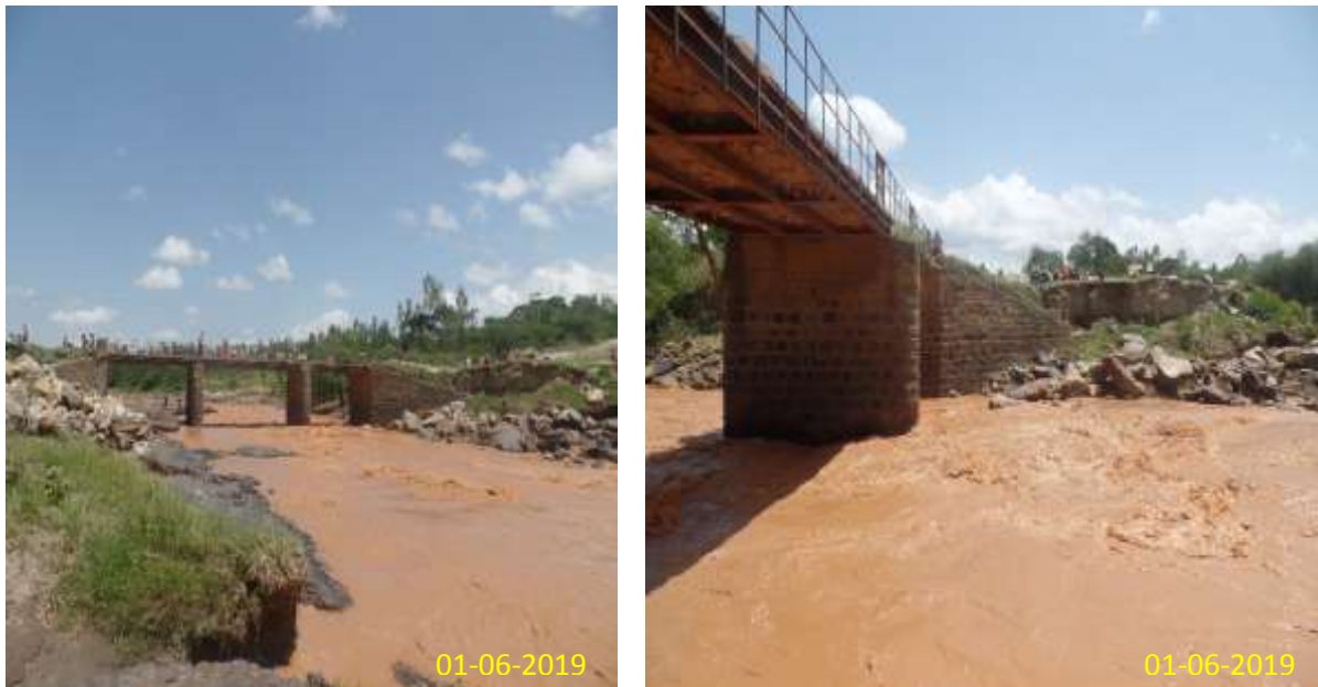
Figure 4.15: Constriction scour effect on the bridge
