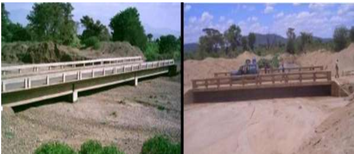
Figure 2.2: Sediment Aggradation on Segen Bridge (Right) and Baso Bridge (Source: (Beza N, 2010))
