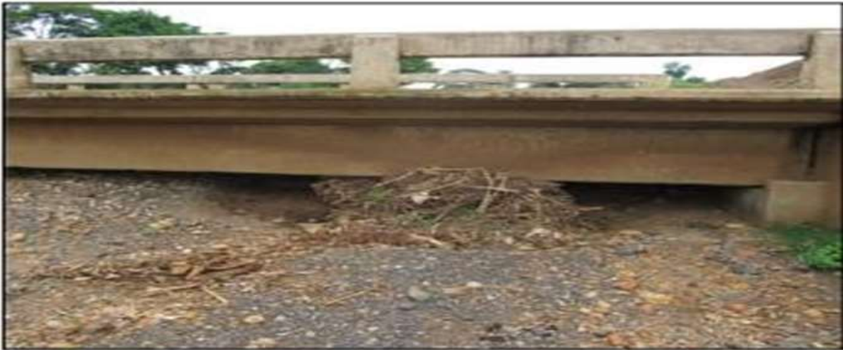
Figure 2.1: Bridge in Arba Minch completely blocked by Debris accumulation
