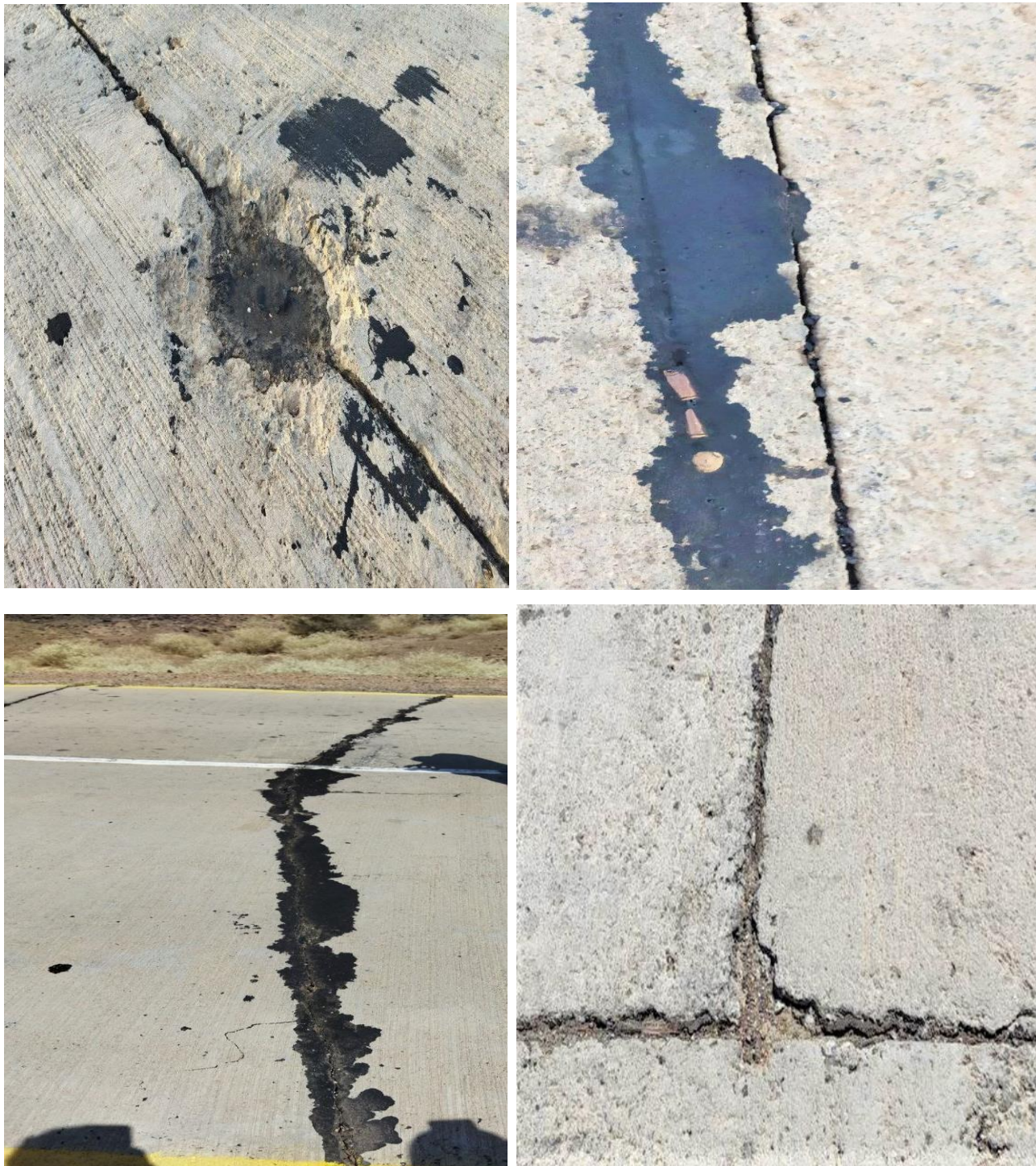
Figure 4.3 Joint sealant failures
