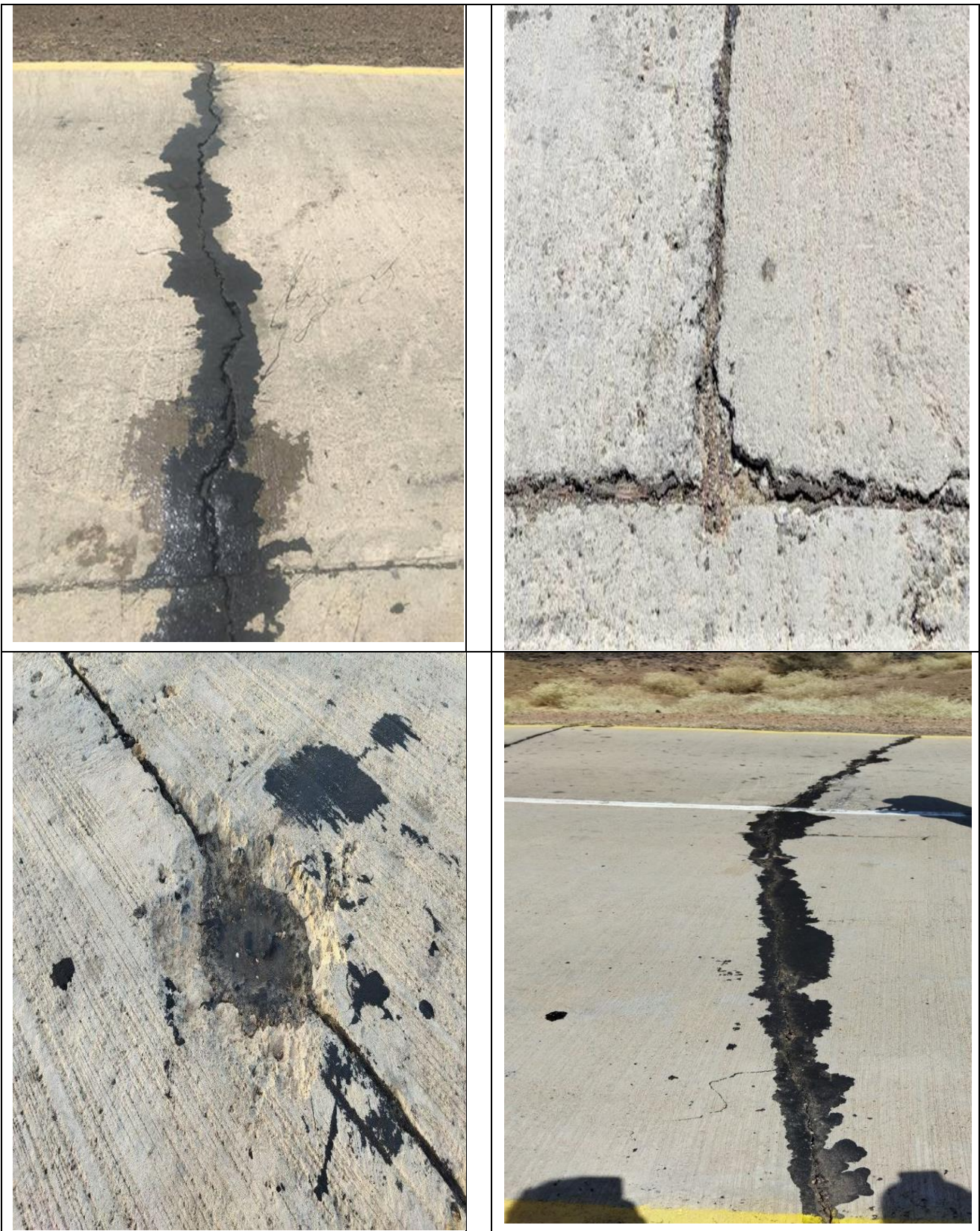
Figure 53. On Ditchoto –Galafi different failure in sealed mixture of Sand and Bitumen
