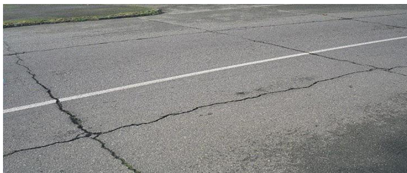
Figure 8. Reflective Cracking ( www.pavementinteractive.org )
