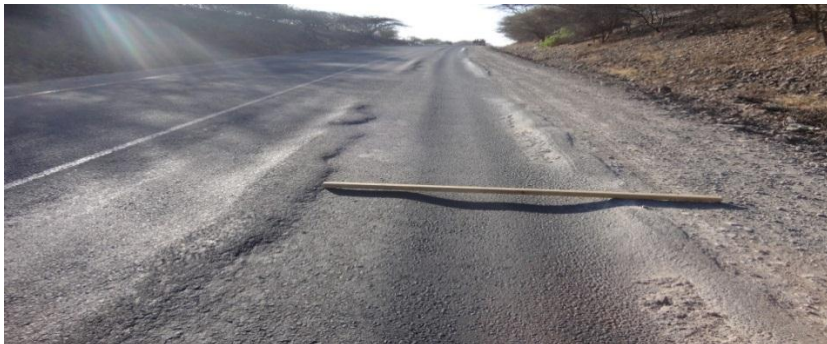
Figure 11. Rutting with Shoving (NET Consult Consulting Engineers and Architects Plc)
