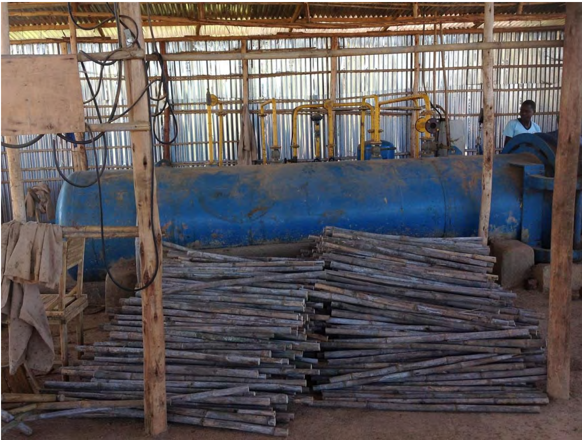
Figure 2-6: Pressurized Chemical Treatment Chamber
