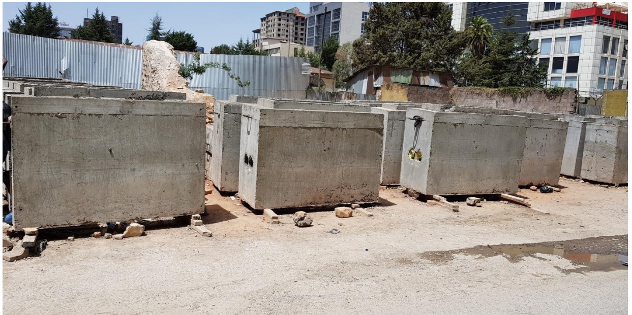
Figure 5. Prefabricated concrete manhole for CBE head quarter project
