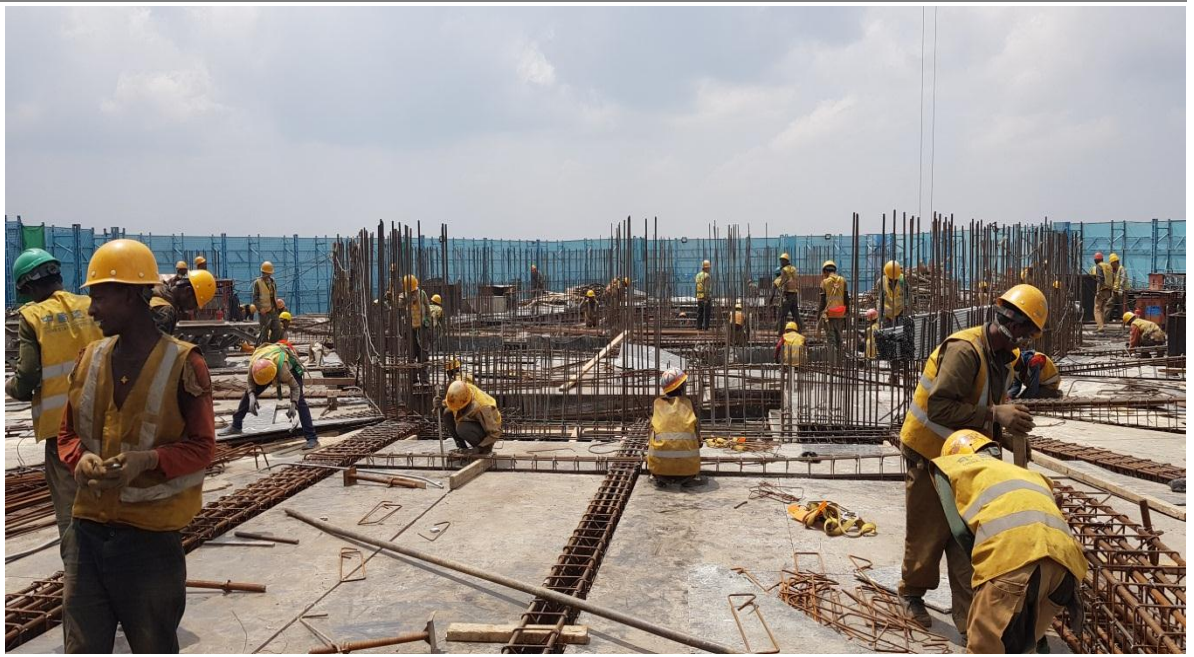
Figure 27 Carpenter and bar bender working on the 30th floor of the tower Starting from this floor the Column isn't composite column simply reinforced concrete column.
