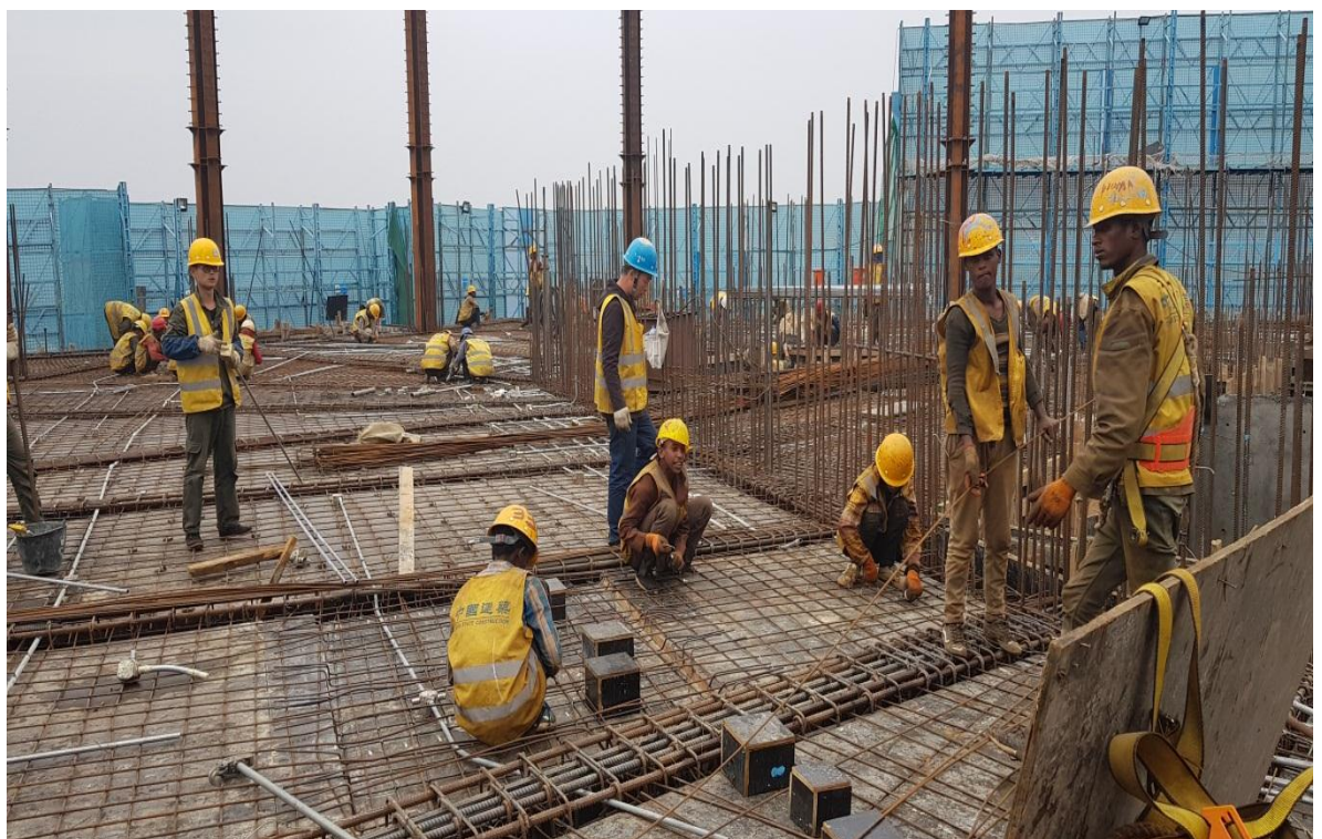
Figure 26 Workers during reinforcement bar & pipe for electric installation fixing on the 29th floor
