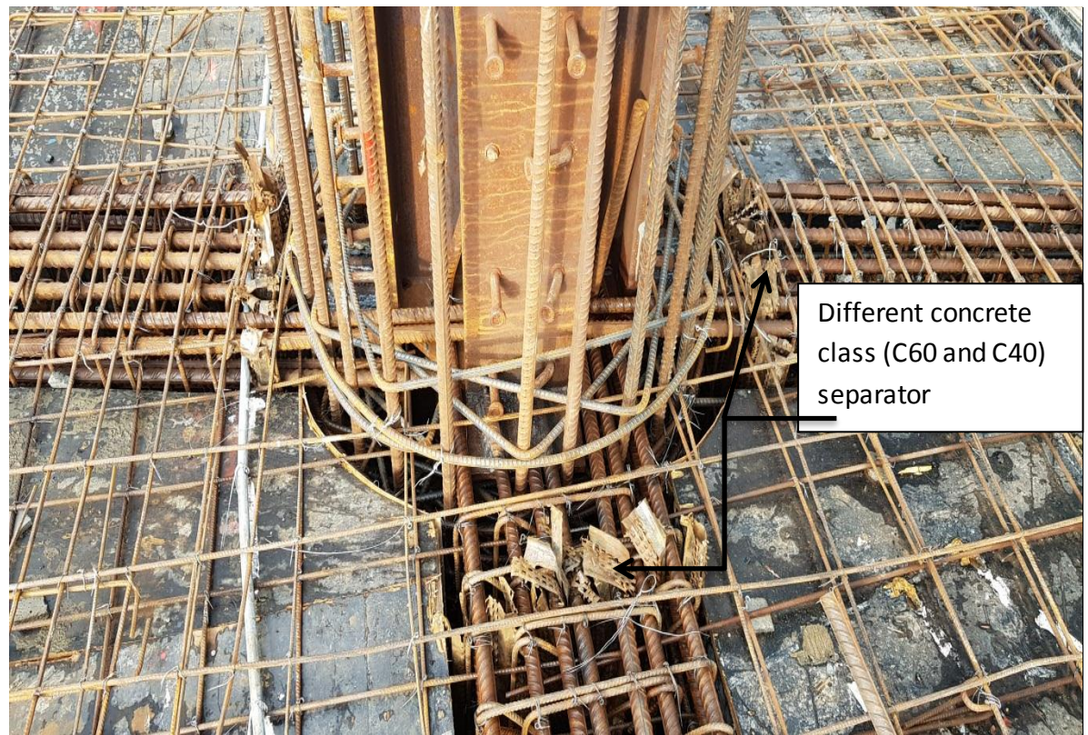
Figure 30 Different class of concrete (for beam & column) separation using rough texture sheet metal
