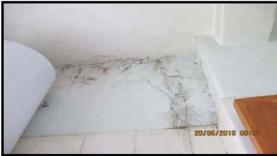
Figure 4.8 Damped wall/slab Surface
