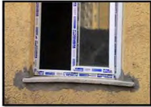
(b) Tilt, improper filings around window frames
