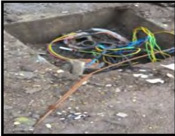
(a) Inadequate protection of electric line
