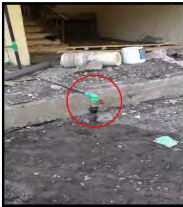
(a) Improper placing of water line
