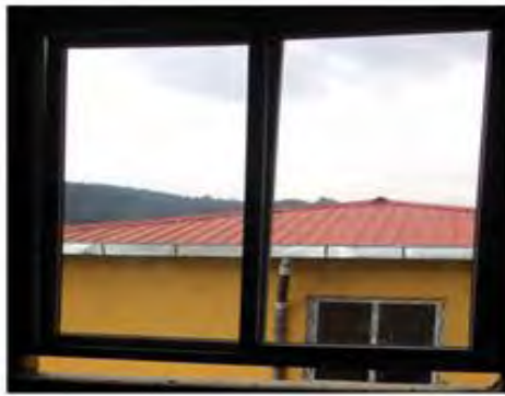
(a) Distorted window frame
