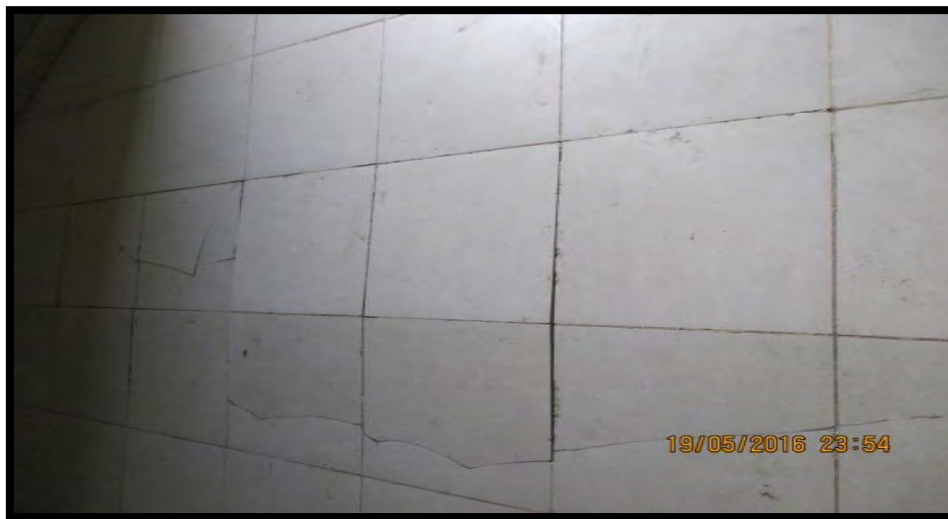
Figure 4.9 Bulged and Cracked Floor /wall Tile
