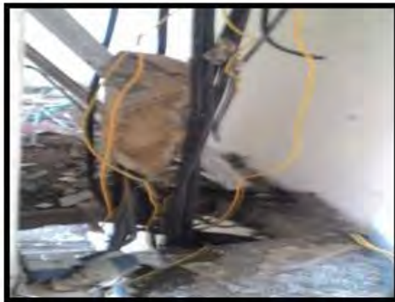
(c) Inappropriate electrical box fixing
