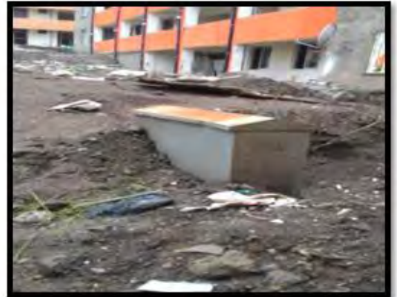
(b) Electric boxes have been corroded
