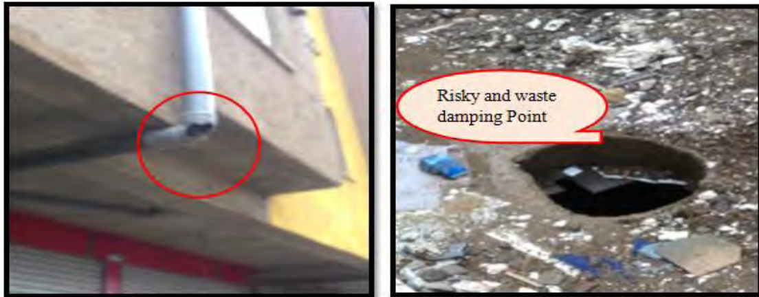
(c) Broken down pipe at the junction
