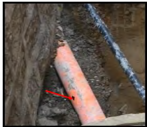
(b) leakage due to broken Sanitary sewer
