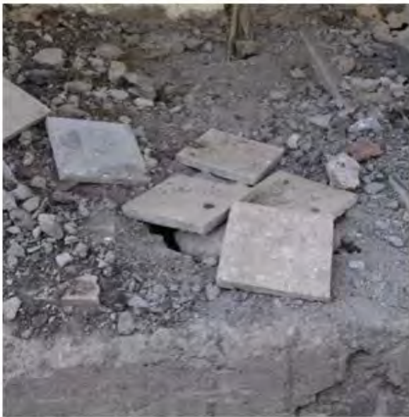
(a) Broken terrazzo tiles
