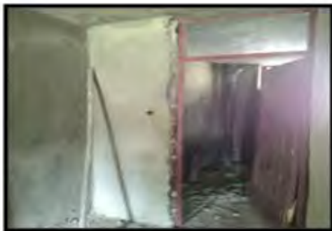
(a) Slanted and poor door fixing
