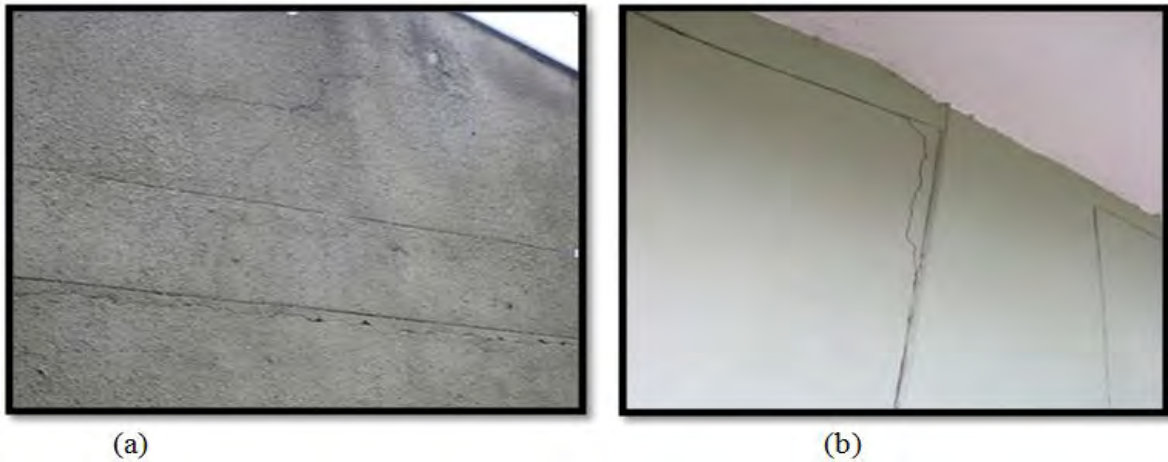
Figure 4.6 (a and b) Diagonal as Well as Horizontal Crack Seen on Walls
