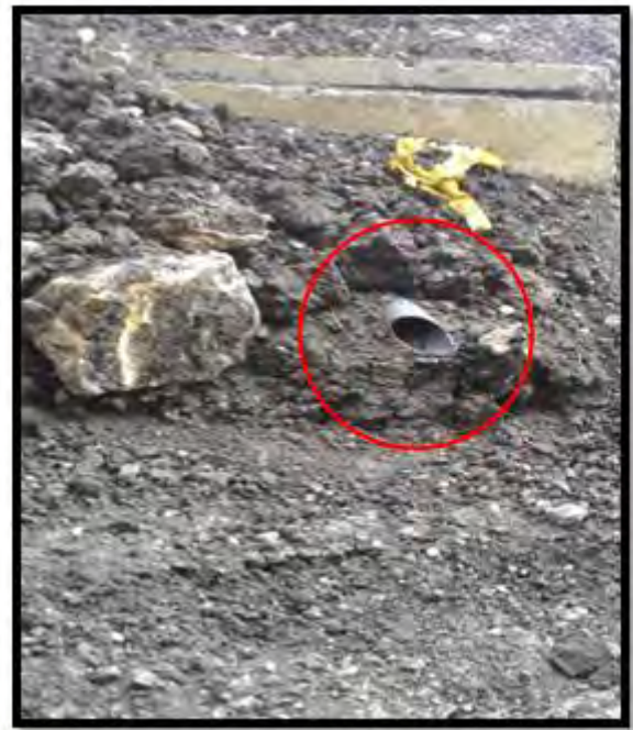
(b) Broken water pipeline
