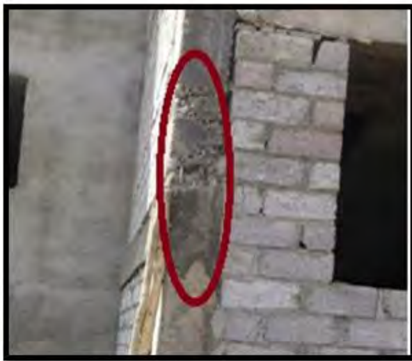
(a) Spill of the concrete cover
