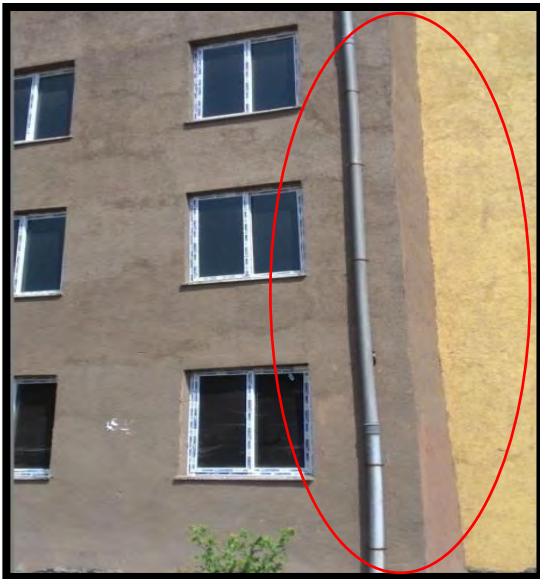
(a) Bulged external wall
