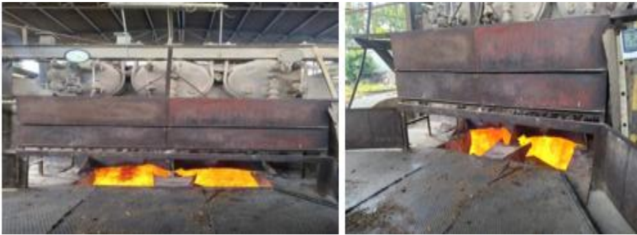
Figure 11: Wood burned at open wood heater: APEPLC
