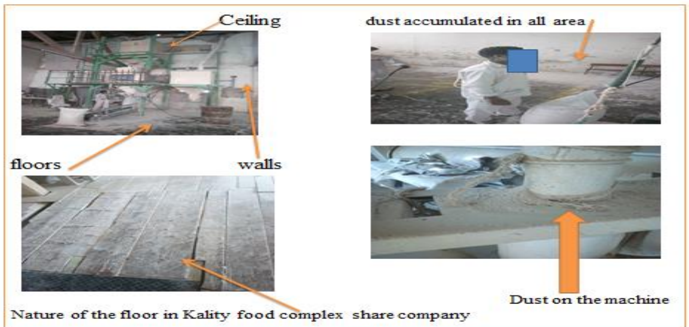
Figure 10: Flour dust accumulated in in different corners of the factories (floor, wall, ceiling and machines of any working sections of the factories, 2019 (By Embay A.)
