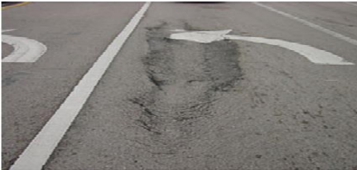
Figure1.0: pavement deform in turning area.
