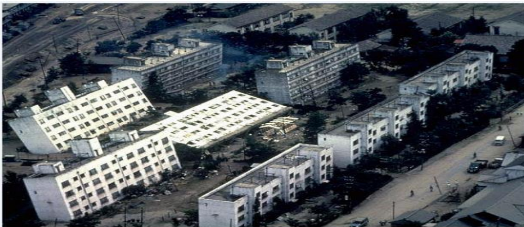
Figure 2-1: Bearing capacity failures caused by liquefaction, after the 1964 Niigata earthquake (source: USGS).
