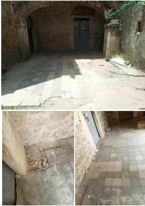
Figure 39. Images showing the floor damages
