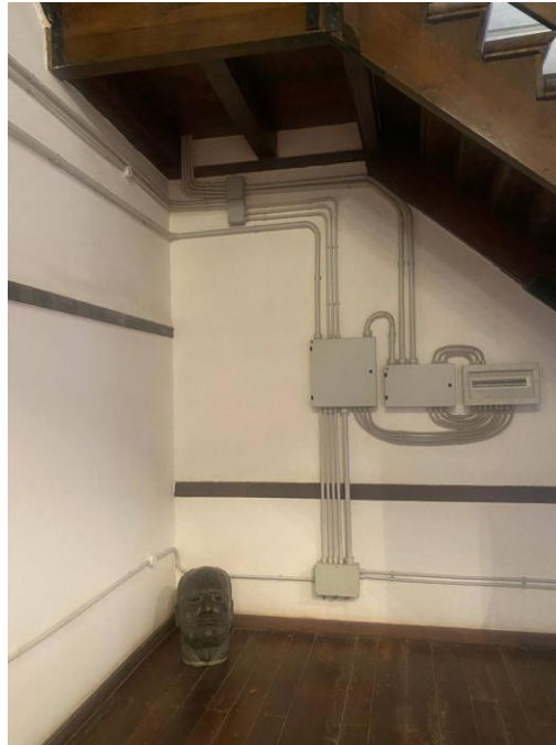
Figure 9. Images showing Atse Yohannes IV Palace electrical installations in the adaptive reused museum
