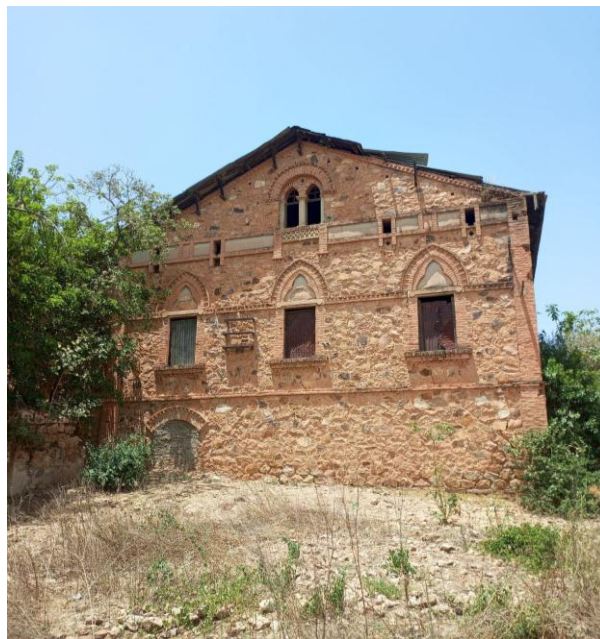
Figure 45. image showing missing windows of the west(left) side of the building
