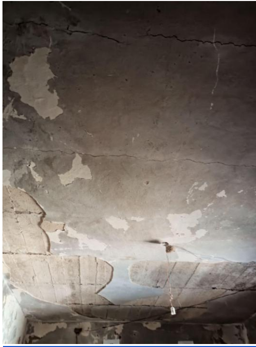
Figure 42. images showing ceiling damages
