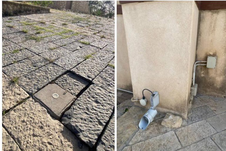
Figure 10. Images showing Atse Yohannes IV Palace pavement and walkway light fixtures installations
