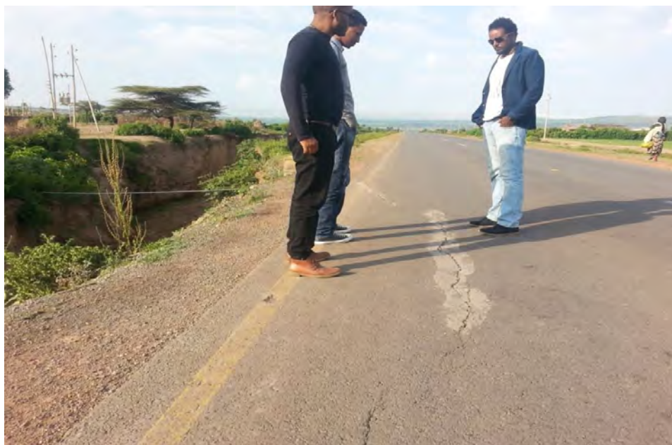
Photo 5.14 Road starts to fail because of erosion gully.
