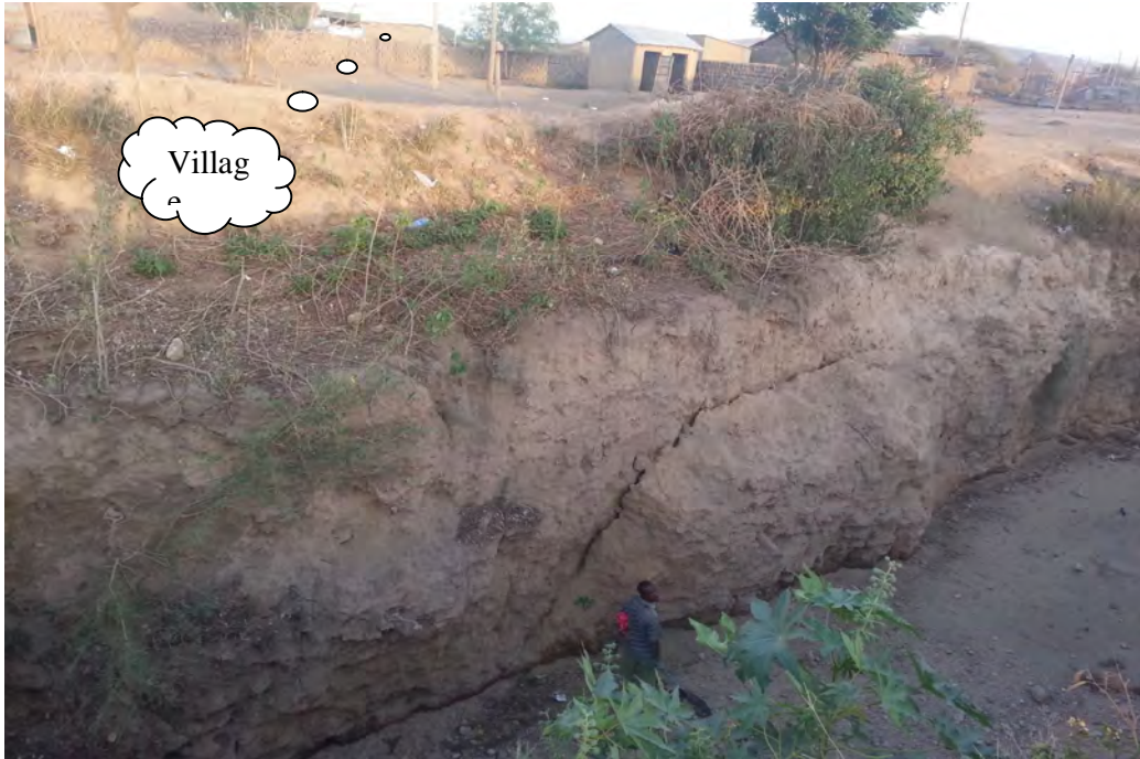
Photo 5.15. Settlement near to the gully area susceptible to land failure.
