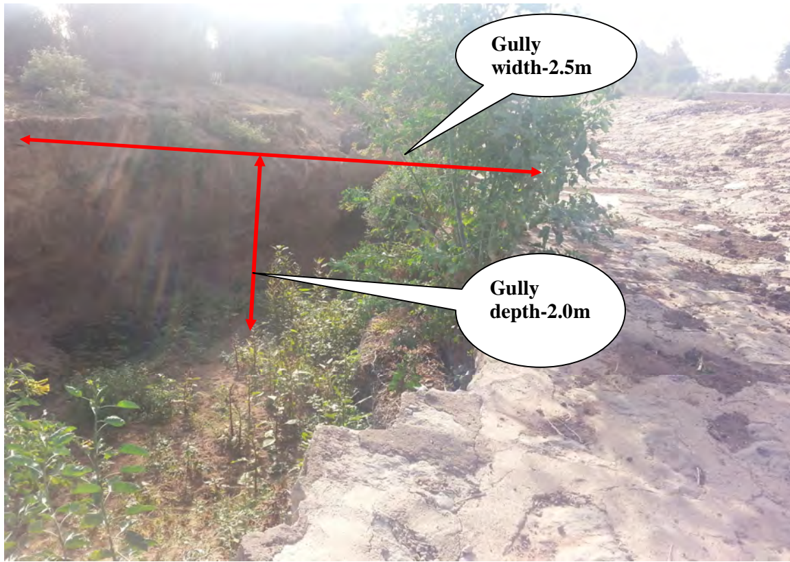
Photo 5.5 Actual condition of erosion gully site -2
