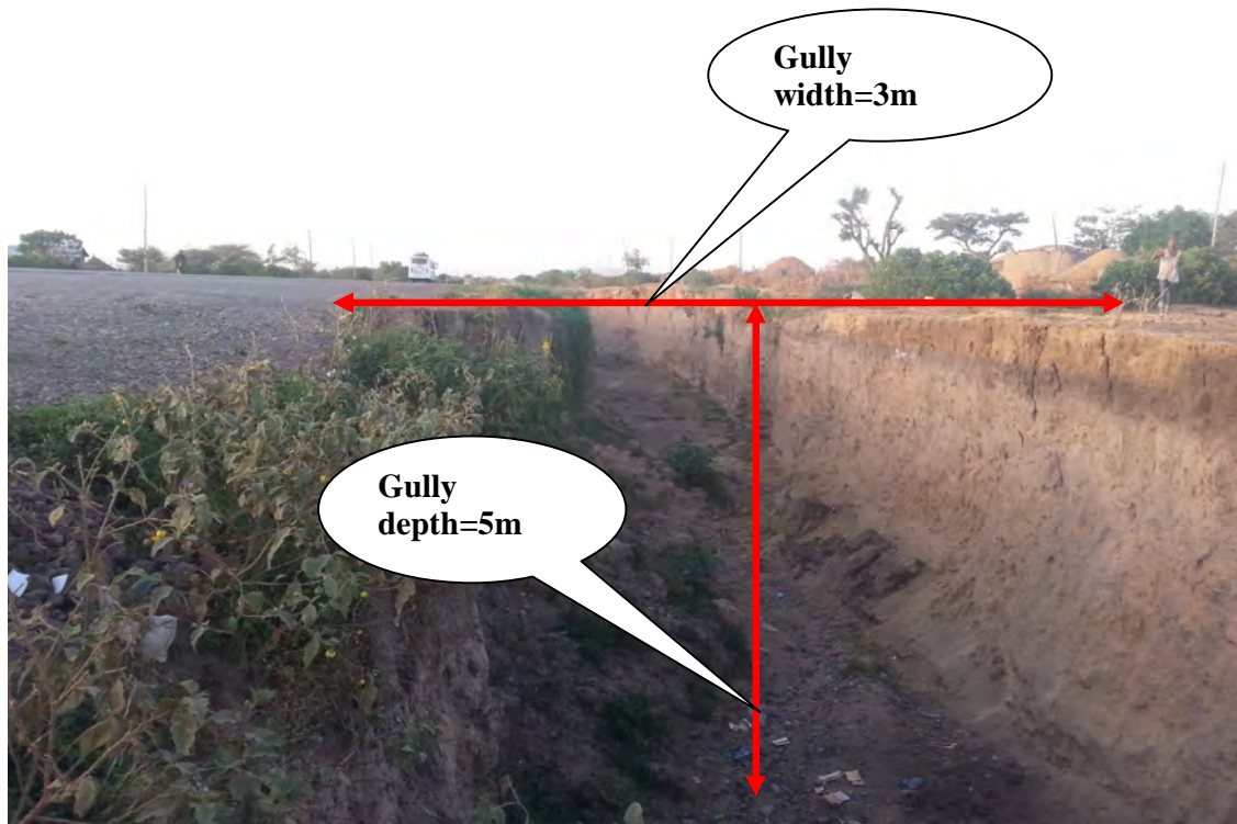
Photo 5.12 Actual condition of erosion gully site-9
