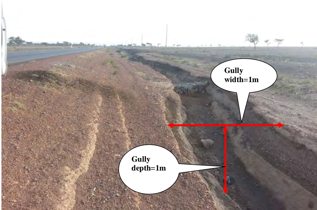
Photo 5.9 Actual condition of erosion gully site-6
