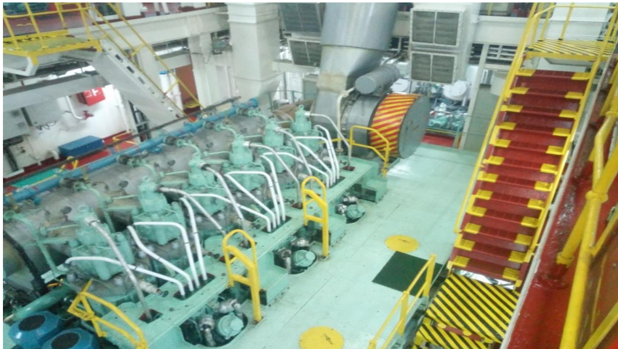
Picture 3-1 Marine Engine system of Marine Vessel Gambella with engine type 6S40ME-B9-TII (Photo Captured by ESLSE Technical officer Bekele Alemu and reprinted with ESLSE permission)
