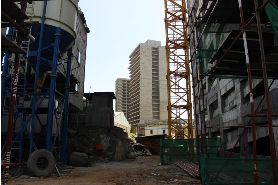
Figure 34: Rear side of ZB-HQP Plot
