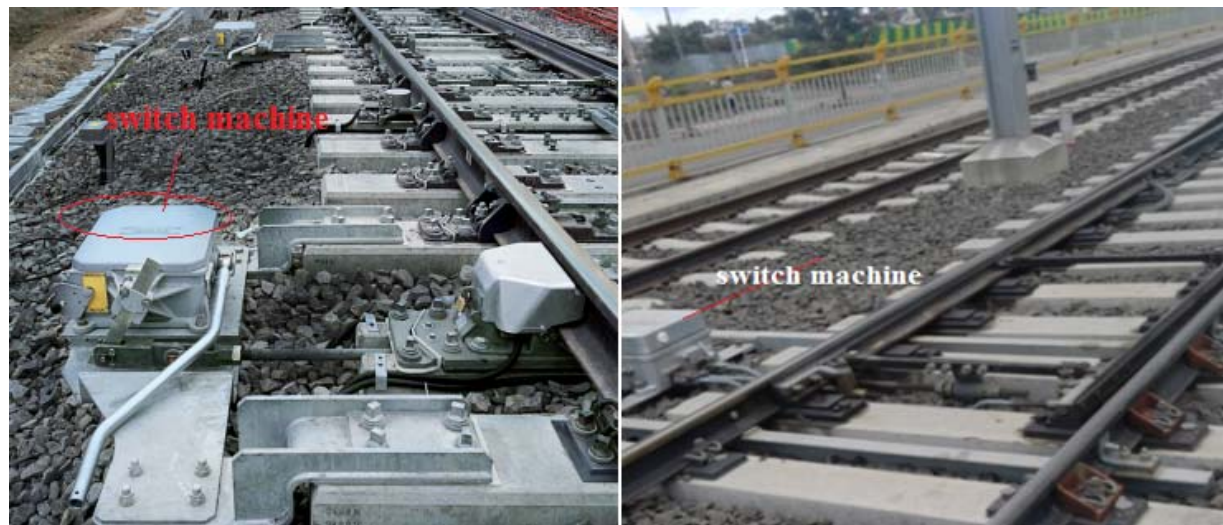
Figure 2.5: Electric switch machine
