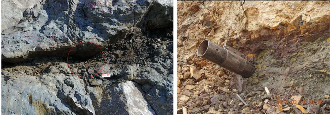
Figure 1.4. (Left) one of J2 joint dipping into \sim 290 with 24 - 30 -degree, filling with thick clay and weathered materials. (Right) in-situ sampling of the J2 infilling material for lab test (Salini-Impregilo, K2 contact characterization, 2017)
