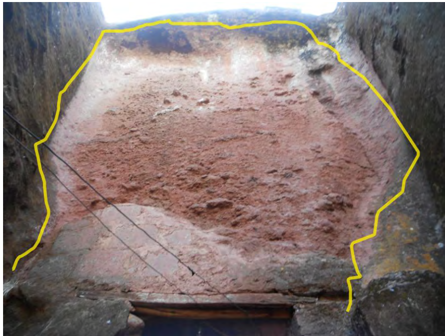
Figure 80: High deterioration of the wall shows here openly at the gate to the courtyard of Bete Ghiorgis, though it is not critically part of the structural elements of the church and it is most probably due to storm rain water and weather effect.
