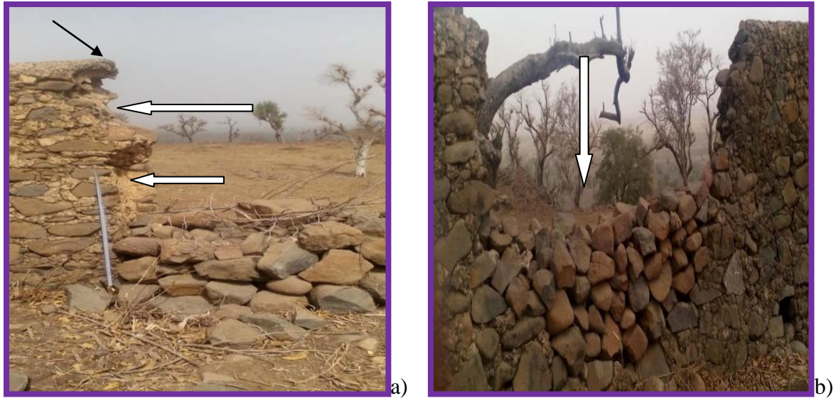
Figure 20: Small gate (a) and damaged part (b) of northern enclosure (Photo by Feyissa H, 2016).
