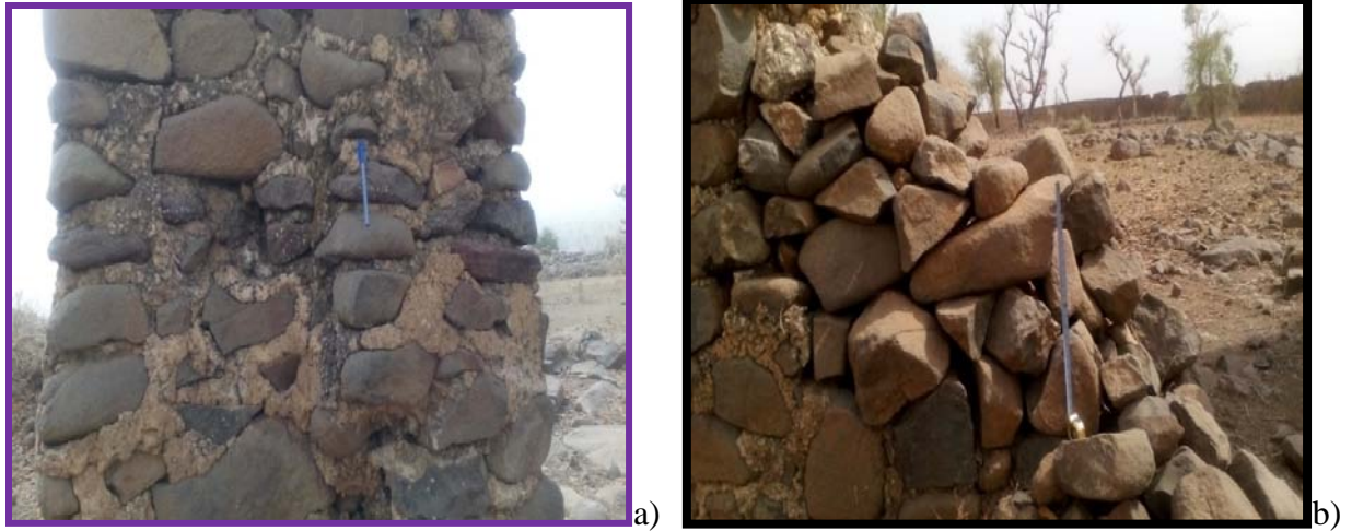
Figure 17: Main gate-intact from eastern side (a) and partly demolished on the western side (b) (Photo by Feyissa H, 2016).
