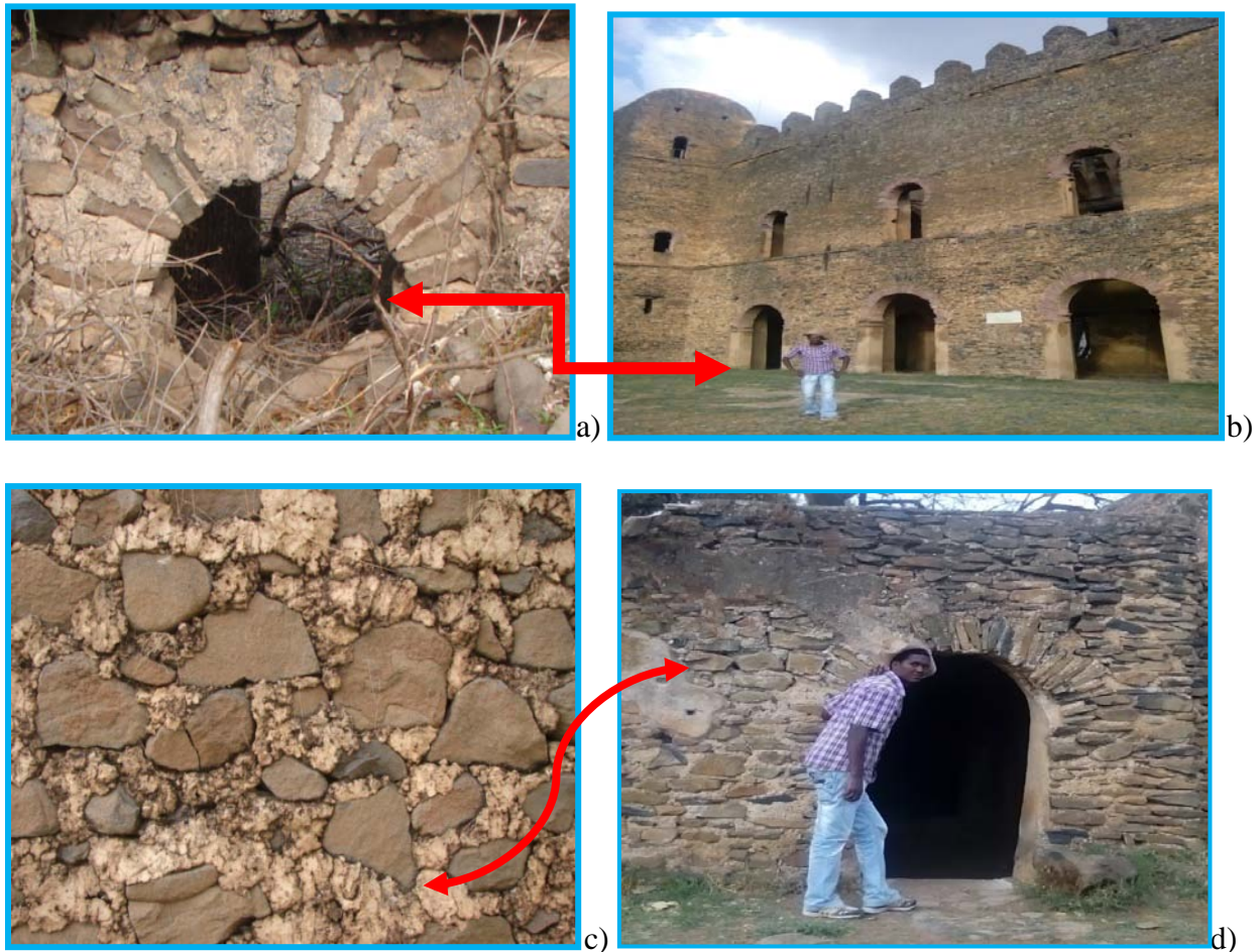
Figure 34: Arch on Bete Mulu castle (a) and on Fasil Ghinb (b), and plastered view of the castle and Ghinb with lime mortar (c) and (d) respectively (Photo by Feyissa H, 2016).
