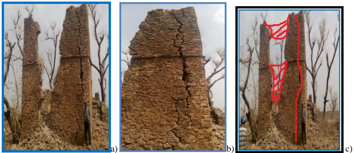
Figure 6: Southern façade of the castle (a), cracking (b), and collapsed (c) (Photo by Feyissa H, 2016).
