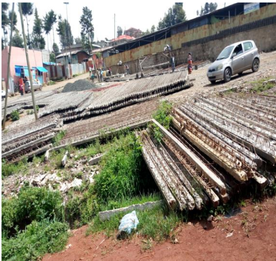
a) Beams stored over the existed public drain.
