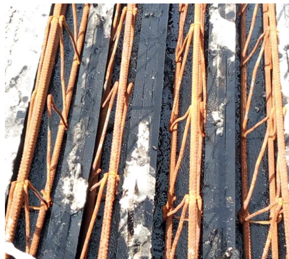
b) Fitting rebars without placing spacer
