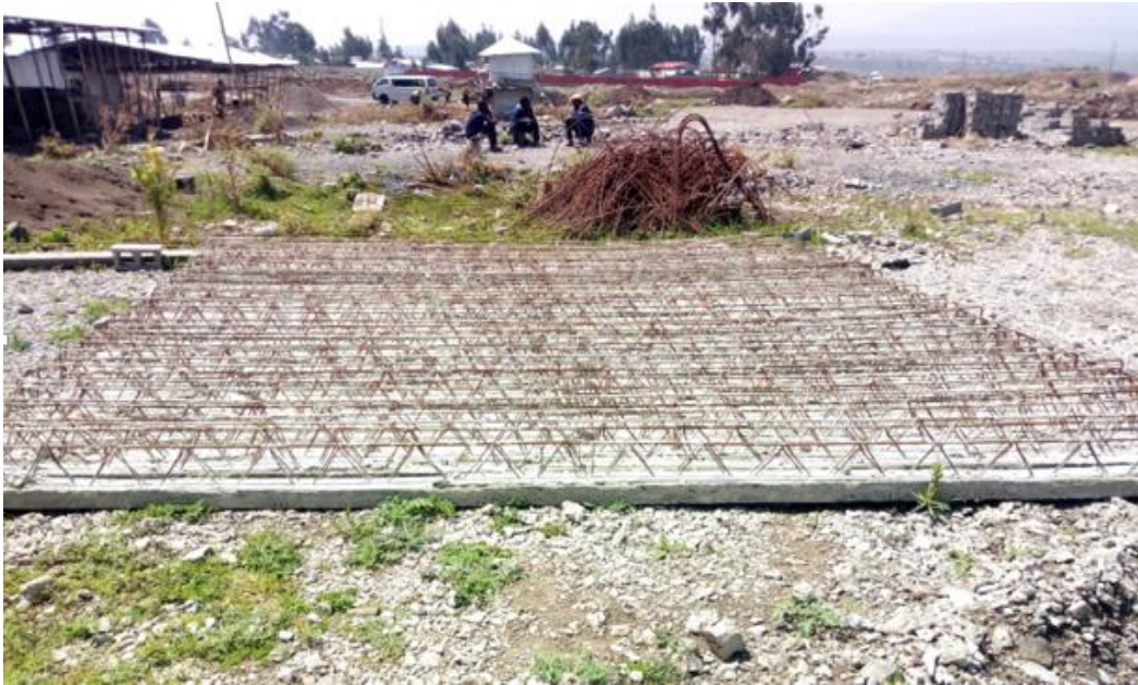
Figure 4.22 The place where ribbed beams cured on the production shade (picture taken by the researcher).
