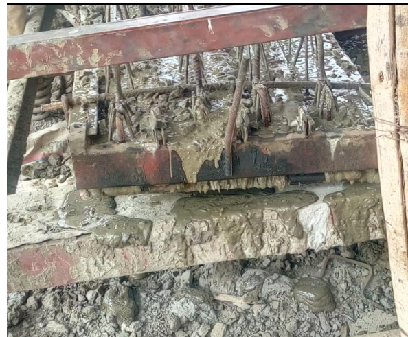
b) Wastes of mortar
