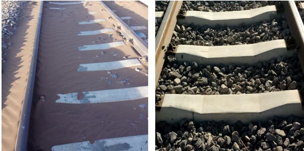
Figure 1.2 Sand Fouled Ballast on the Left (Adigala) on Ethio-Djibouti Line and Clean Ballast on the Right.
