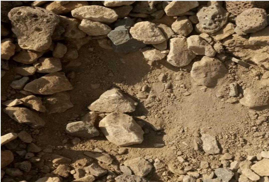
Figure 3.4 Fouled Ballast During Sample Excavation
