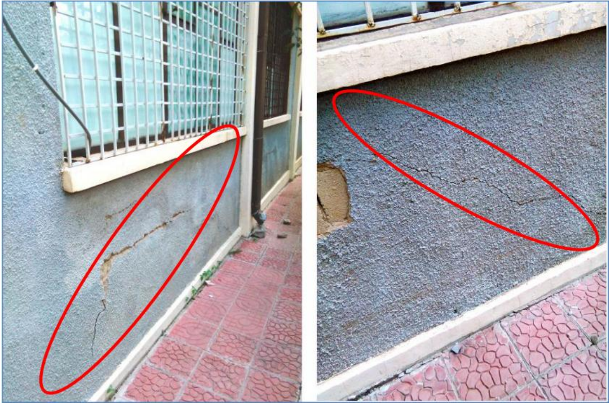
Figure 3.5 Infill walls diagonal cracks along the Axis C
