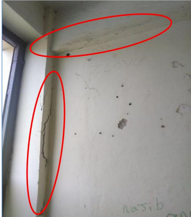
Figure 3.7 Along axis C column crack
