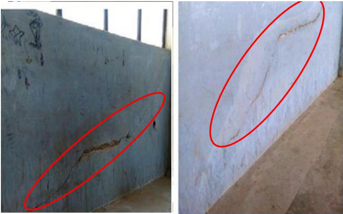
Figure 3.4 Internal infill walls diagonal cracks along Axis B
