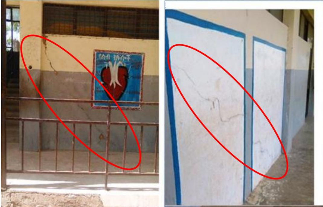
Figure 3.3 External infill walls diagonal cracks along Axis B
