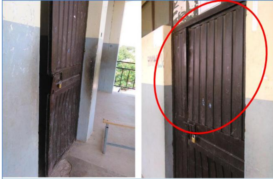
Figure 3.9 Building's steel doors distortion
