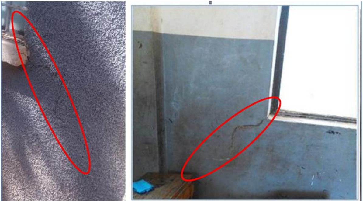
Figure 3.6 External and internal side's window corner diagonal cracks
