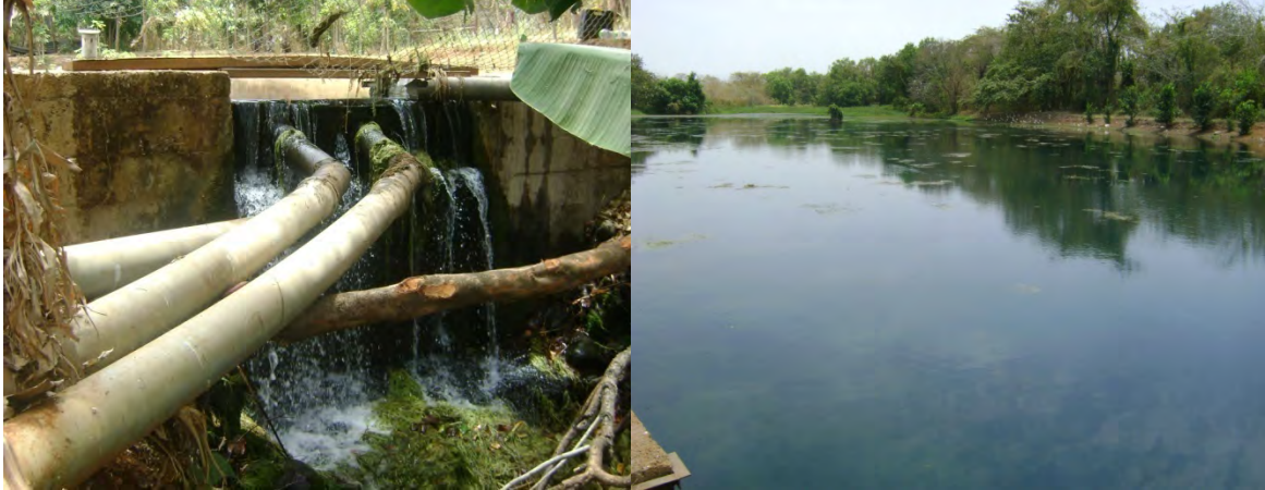
Plate3.2 Ali spring. The left hand side picture is the spring over flow, with non functional irrigation pipelines. The right side is the dam from the spring.
