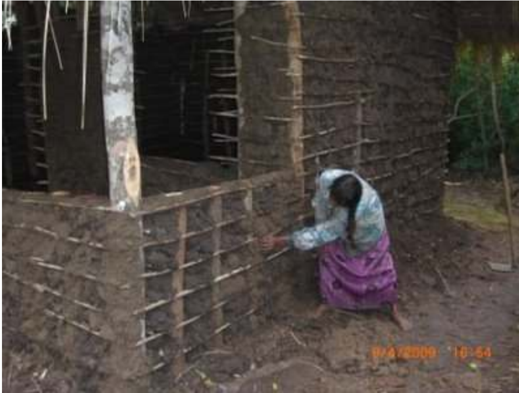
Fig.3.4 Mud covering on bamboo wattle wall [29]
