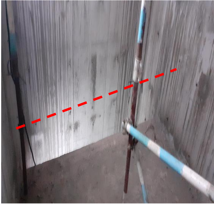
No riser on barricade shaft opening
