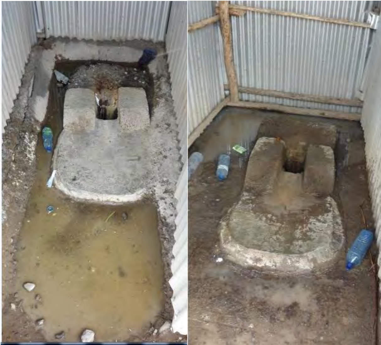
Figure 5: A sample photo of latrine used by the trainee with full of dirty overflowing sewage and without slap.
