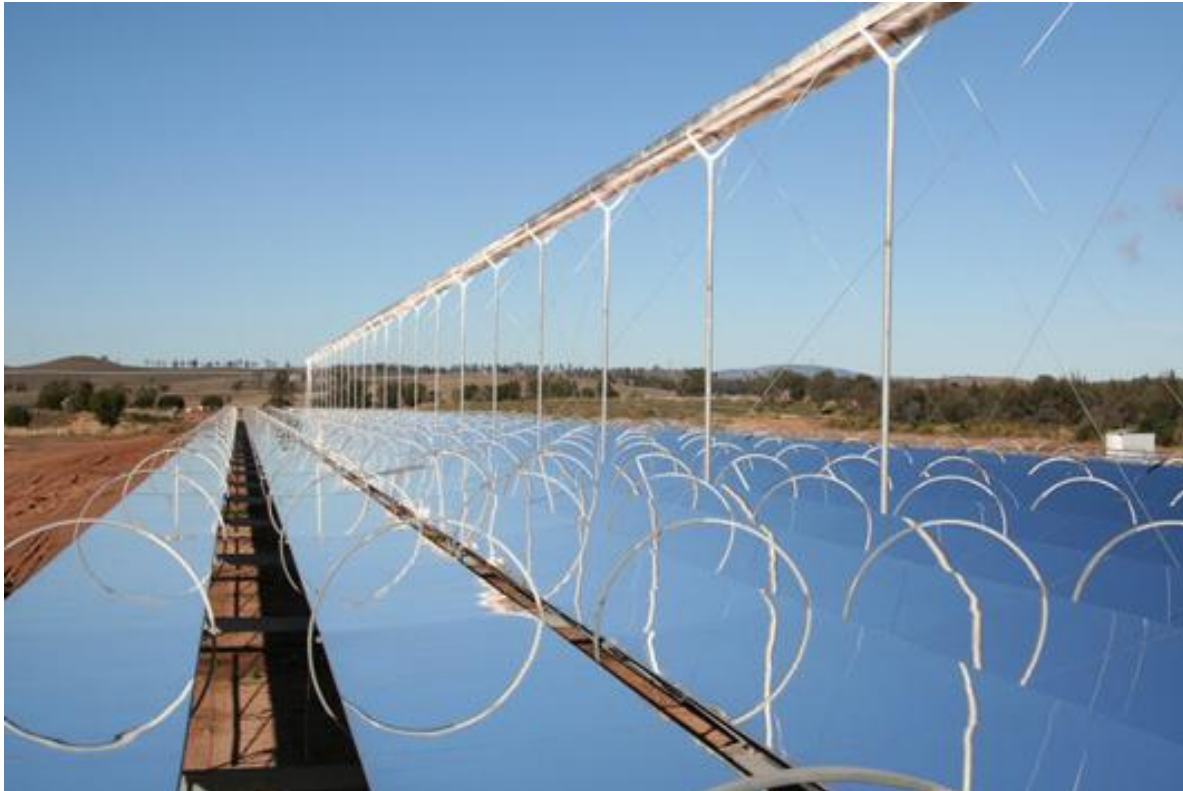
Figure 1-4: Compact Linear Fresnel Collector in Bakersfield, California by Ausra
