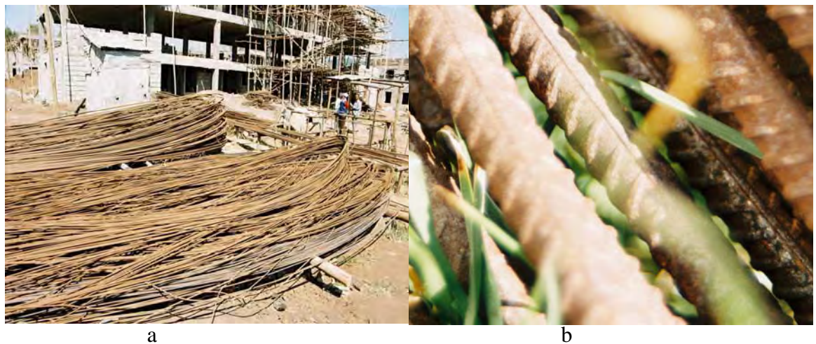
Fig. 2.3 Rusting of Reinforcement Bars
