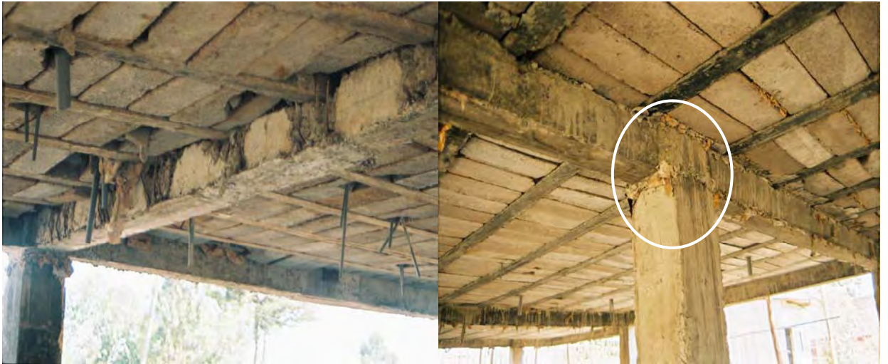
Fig. 2.4 Defects Due to Poor Workmanship
