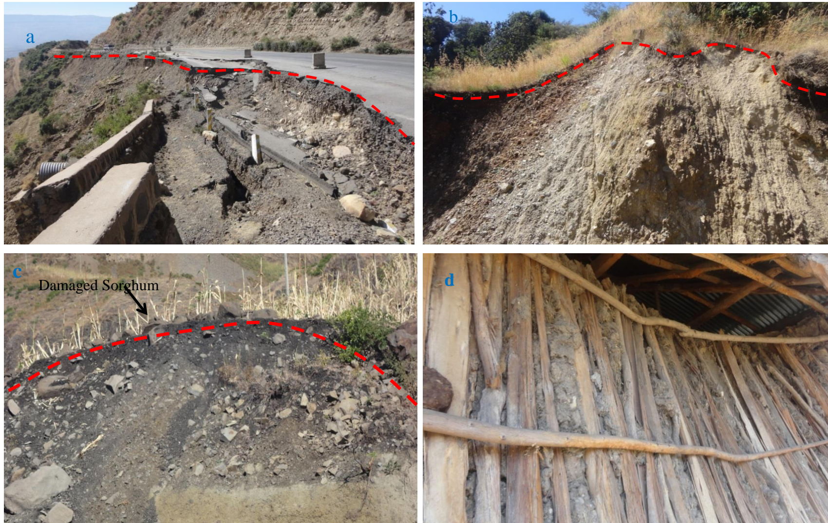
Figure 1.3 Field photos illustrating landslide problem a) completely damaged road; b) damaged grass land and soil; c) destructive agricultural land with sorghum and d) completely damaged local home
