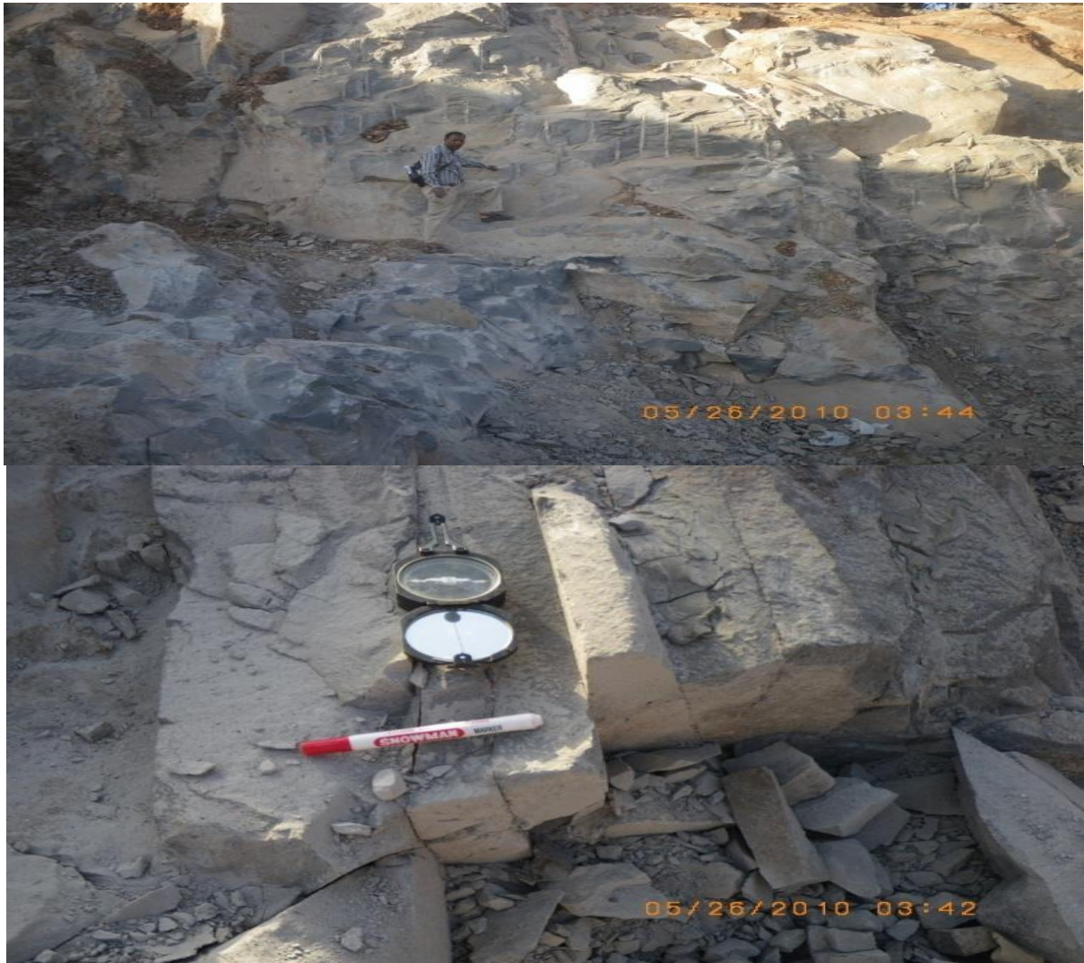
Plate 1.4: NE-SW oriented discontinuities (sub-parallel to the regional structures), encountered on massive basaltic intrusions. It was exposed during excavations in a ring road construction project, Adissu Gebeya, AA.
