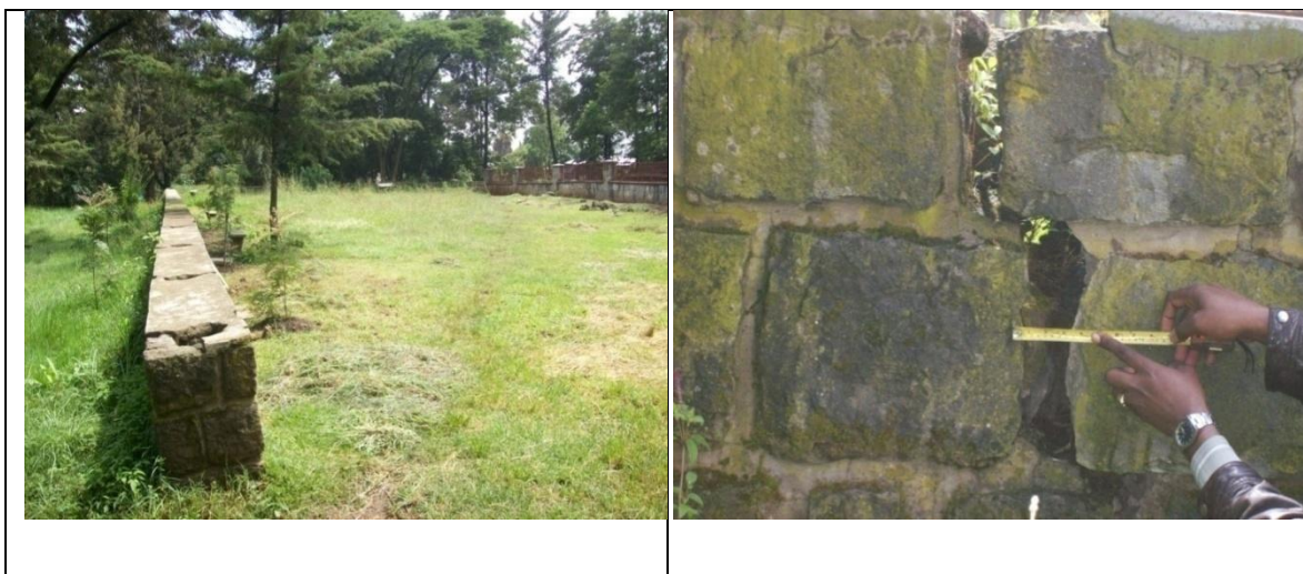
Plate 4.6 Displaced infrastructures due to landslide problem: a ground tennis court in Yeka Park, Addis Ababa has been found displaced east wards. As measured by measuring tape, the retaining wall has moved apart a distance of about 20cm.
