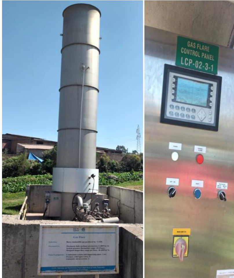
Figure 1.3 Existing Biogas Flare System
