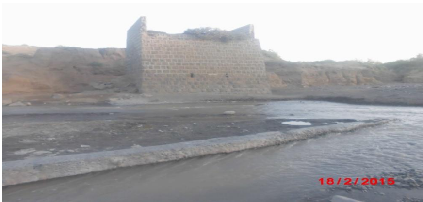
Plat 6.5 uwa river showing bridge collapses because of flood in summer time.
